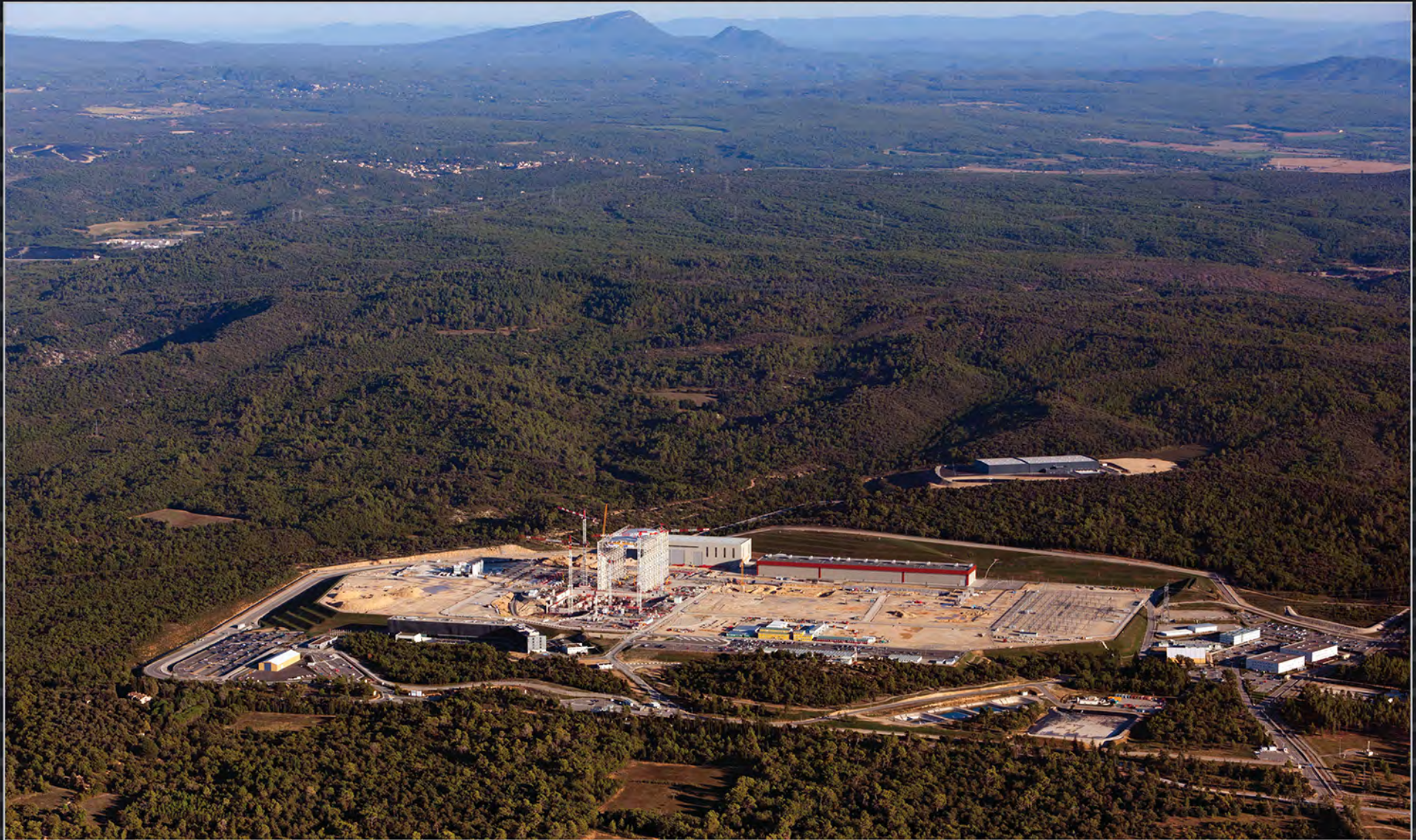
A little over half of the "ITER parcel" has been cleared – the rest remains wooded. Behind the platform, a 9,000 m 2 warehouse is now in place for the storage of delivered components. September 2015
