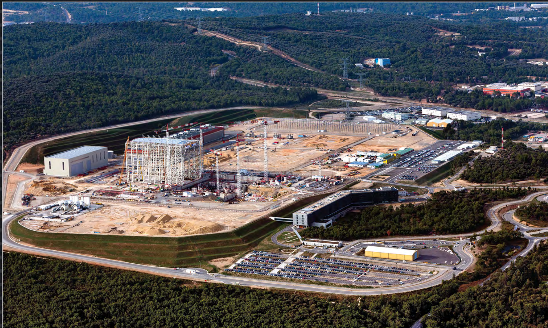
Since the completion of its metal structure the Assembly Building is the tallest building on the ITER platform, rising 60 metres above ground level. Here pre-assembly activities will be carried out on the principal tokamak components prior to machine installation. September 2015
