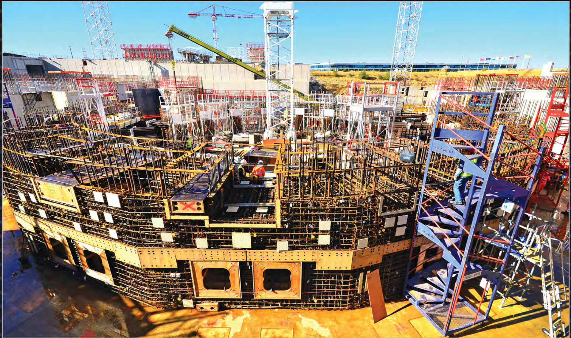
The 3.2-metre-thick ITER bioshield will completely enclose the ITER Tokamak and its cryostat. In the dense reinforcement set into place in advance of concrete pouring, openings are visible for the arrival of electrical and cryogenic supplies.
