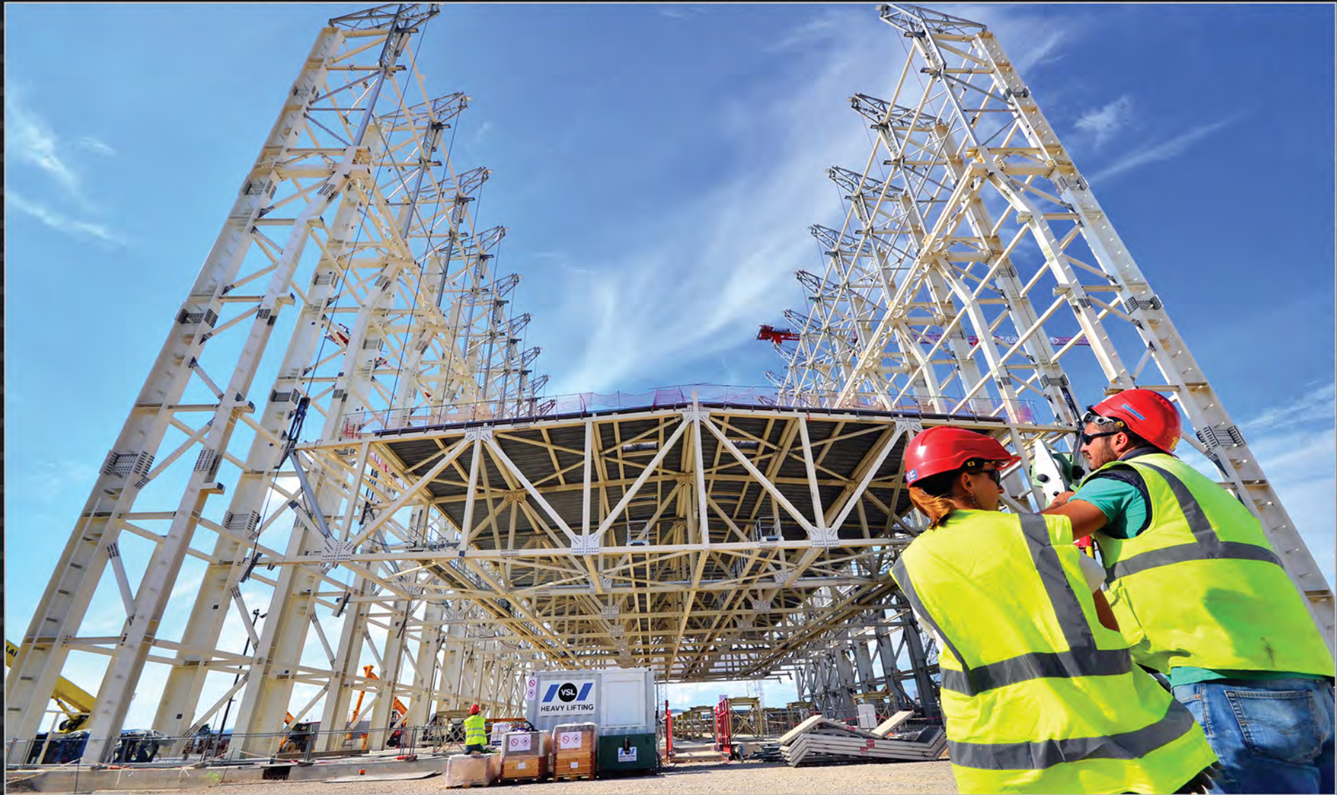
In a carefully programmed operation that lasts 14 hours, the 730-tonne roof structure of the Assembly Building is successfully lifted into place. Now, the building can be fitted out with exterior cladding and rails for the heavy-lift cranes. September 2015
