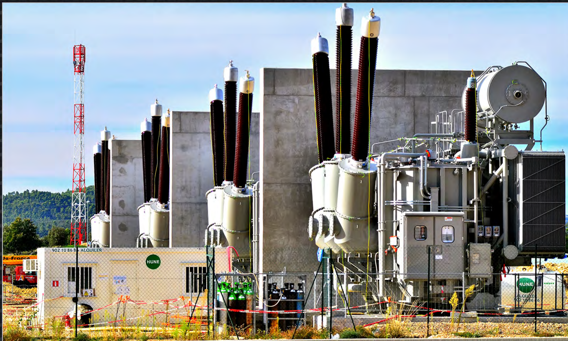
Four US-supplied high voltage transformers were the first plant components installed at the ITER site in September 2015. The US also completed delivery of 22 kV switchgear components to the European Union for the steady state electrical network.
