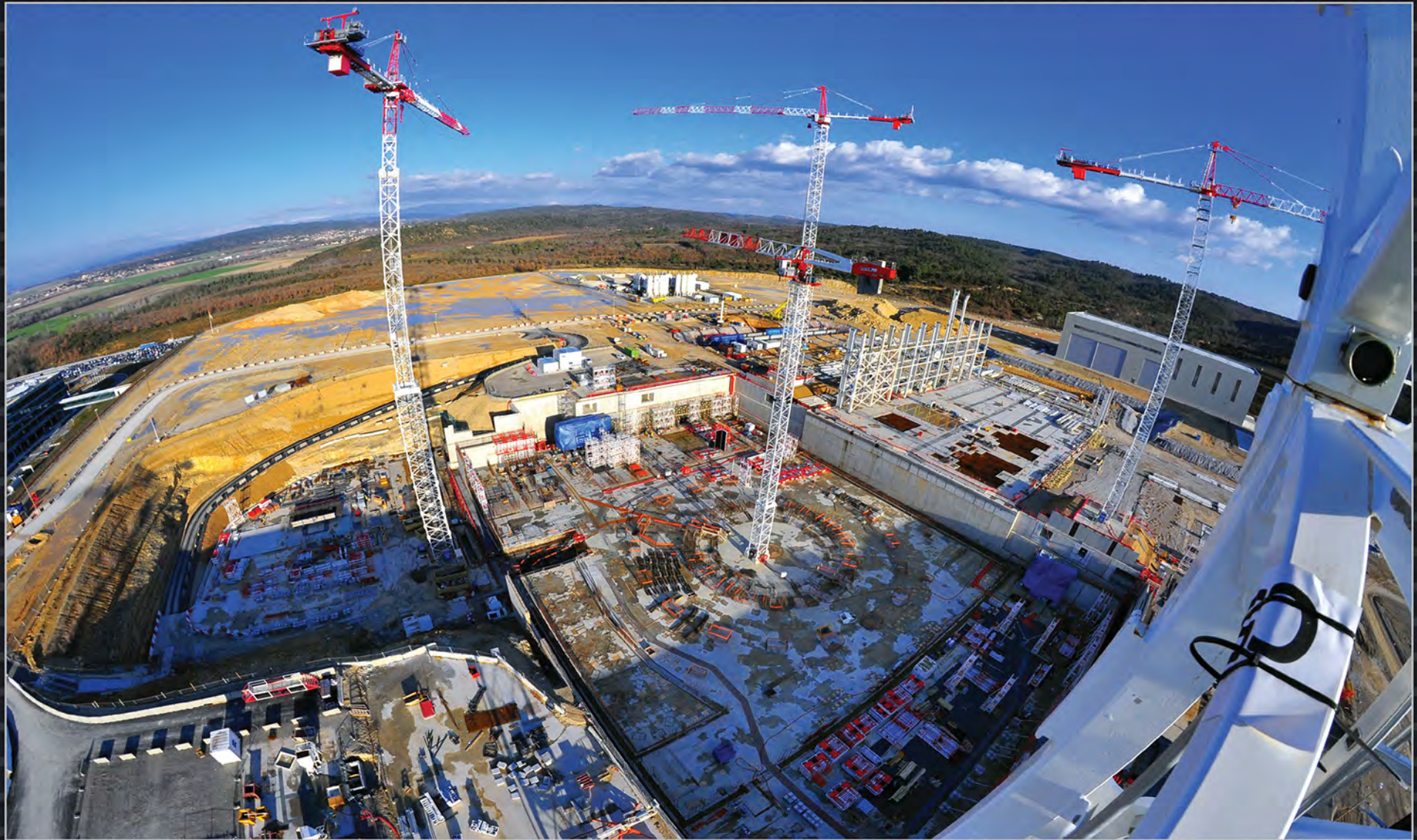
Work is underway on the lowest basement level (B2) of the seven-storey Tokamak Complex. To the east, the first pillars of the Assembly Hall are visible. February 2015
