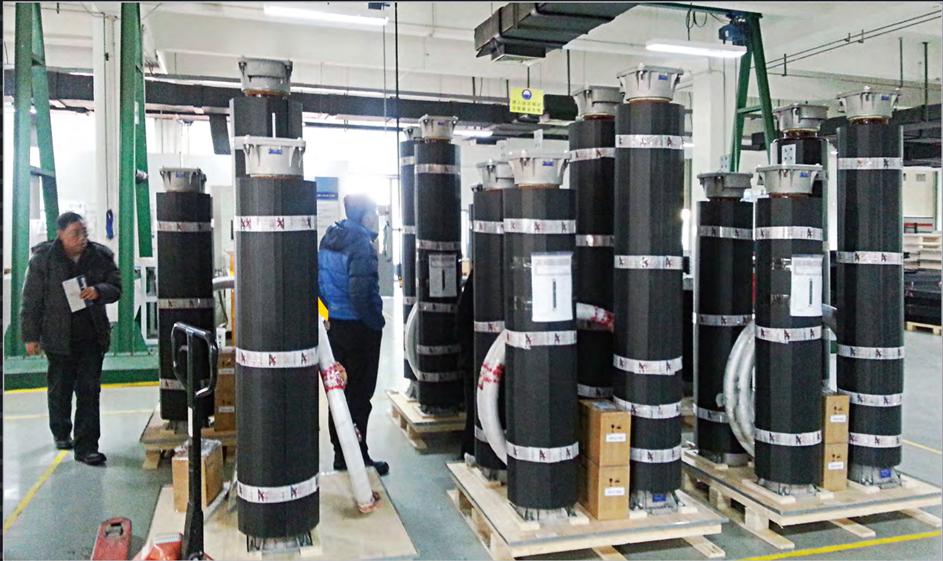
The pulsed power electrical network (PPEN) provides power to the "pulsed" systems of ITER, including the magnet power supplies and plasma heating systems. A first batch of PPEN equipment (surge arresters, current transformers, potential transformers, disconnecting switches and earthing switches) has been manufactured and tested in China, and is now ready for shipment.
