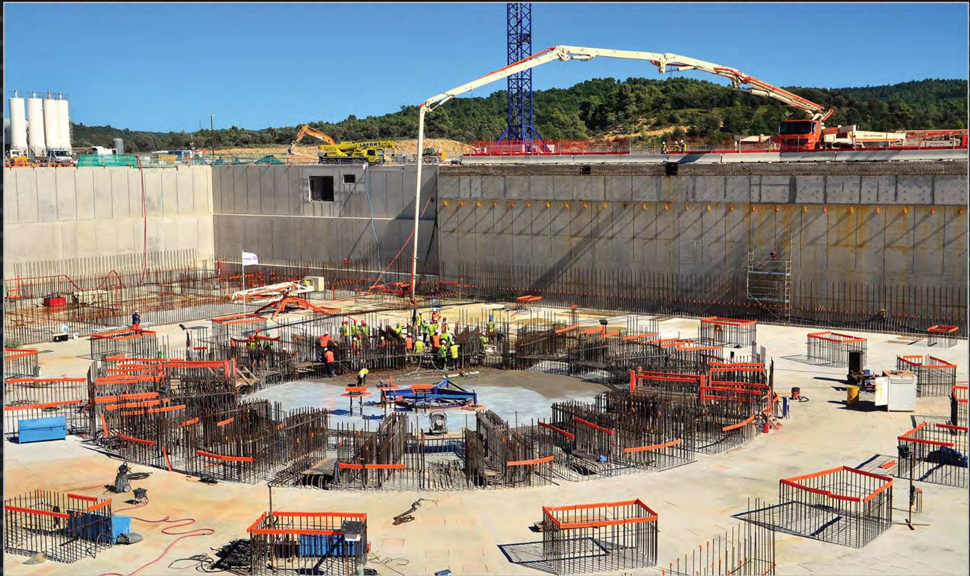
Four years of work in the Tokamak Pit to create the ground support structure and foundations of the Tokamak Complex are brought to a successful conclusion as the last segment of the B2 slab – the basemat that will support the machine and systems – is poured. August 2014
