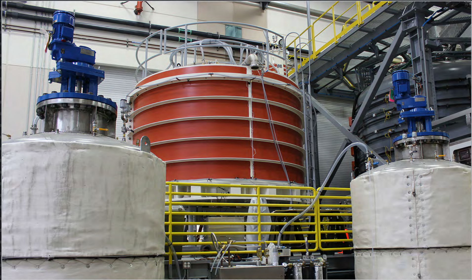
The central solenoid vacuum pressure impregnation station has been installed. The station will inject an insulating epoxy mixture around the modules.
