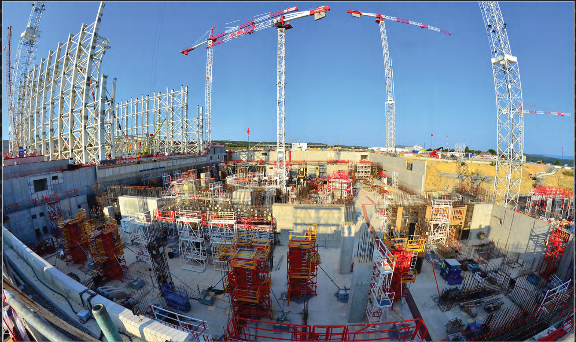
Work progresses in 2015 on the columns and walls of the first basement level (B2) of the Tokamak Complex. At the same time, the metal structure of the giant Assembly Hall takes shape. July 2015
