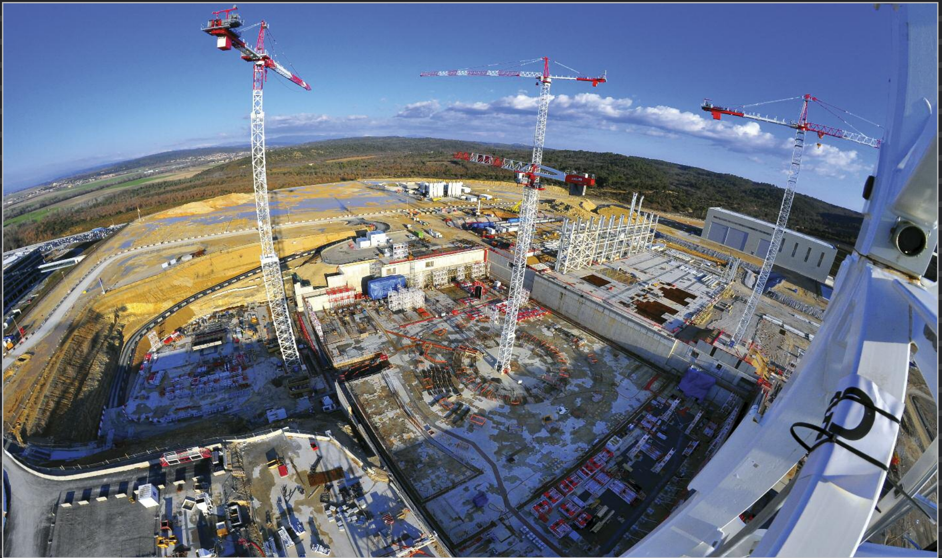
Work is underway on the lowest basement level (B2) of the seven-storey Tokamak Complex. To the east, the first pillars of the Assembly Hall are visible.
