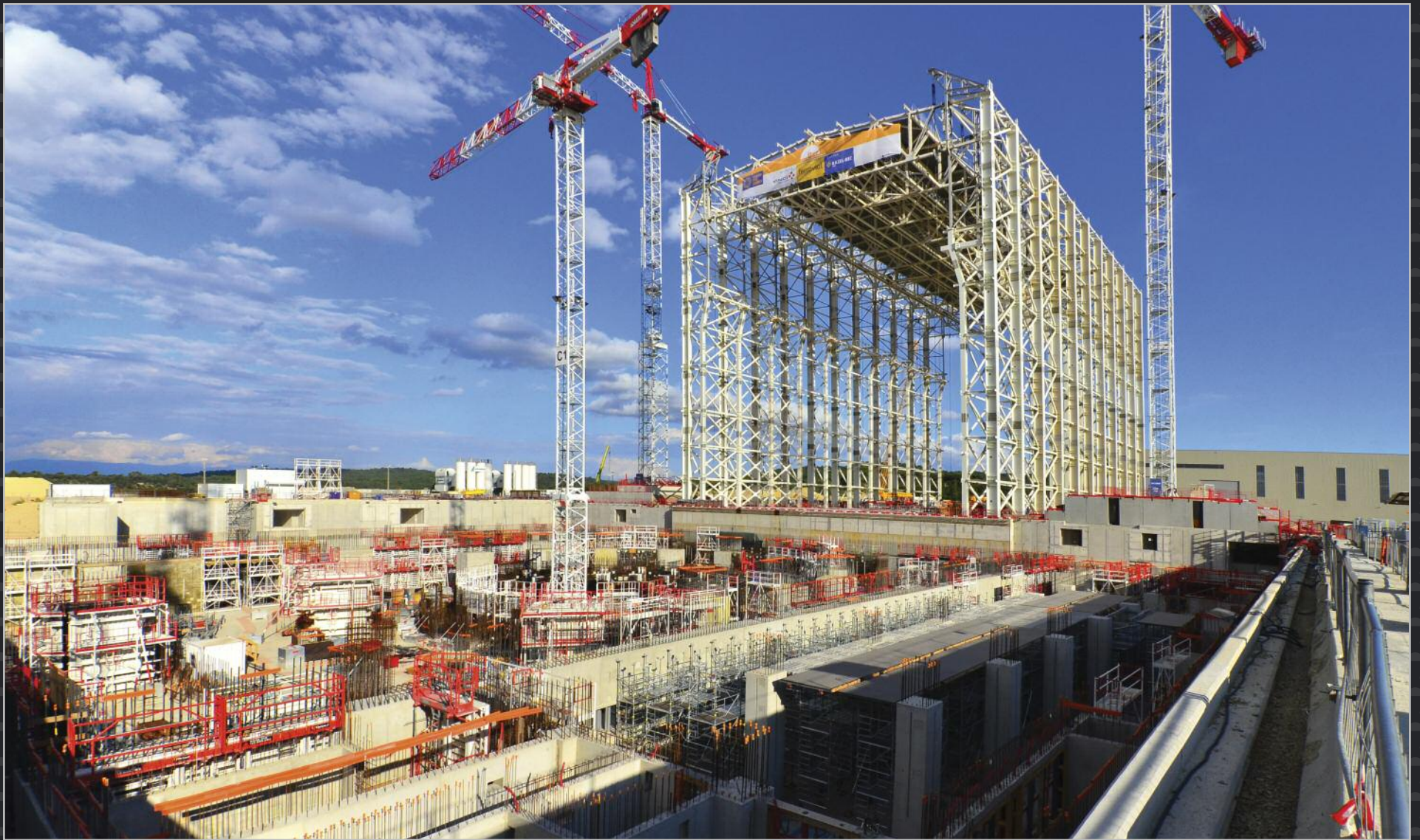
When completed, the Tokamak Building (under construction, in the centre of the basemat) will be as tall as the just-topped Assembly Building. September 2015
