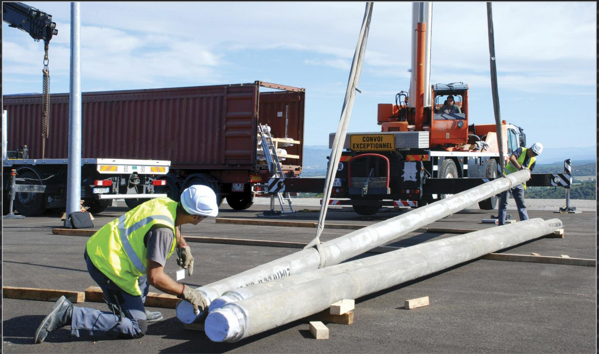
The first cooling water piping under Indian scope reaches ITER in September 2015. In all, India will ship 100 containers of piping for ITER's chilled water and heat rejection systems.
