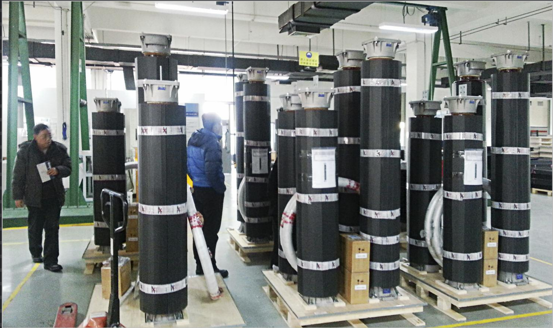
The pulsed power electrical network (PPEN) provides power to the "pulsed" systems of ITER, including the magnet power supplies and plasma heating systems. A first batch of PPEN equipment (surge arresters, current transformers, potential transformers, disconnecting switches and earthing switches) has been manufactured and tested in China, and is now ready for shipment.
