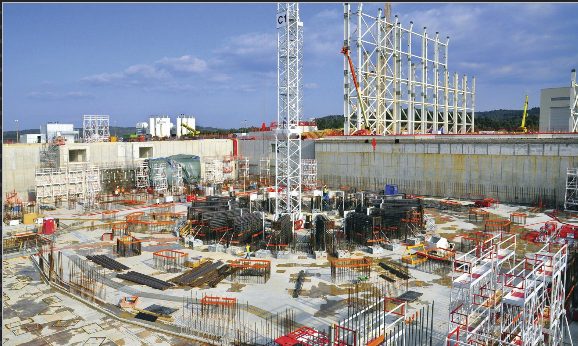
Eighteen radial structures will link the cryostat support “crown” to the surrounding concrete bioshield, helping to distribute the considerable force that will be exerted by the combined mass of the machine and the cryostat (25,000 tonnes) as well as structural movement. March 2015
