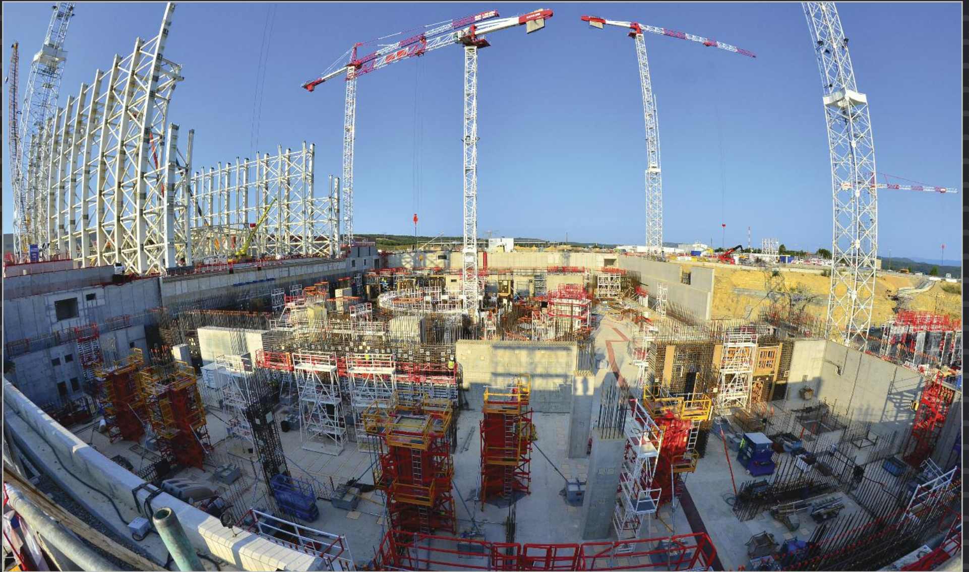
Work progresses in 2015 on the columns and walls of the first basement level (B2) of the Tokamak Complex. At the same time, the metal structure of the giant Assembly Hall takes shape. July 2015
