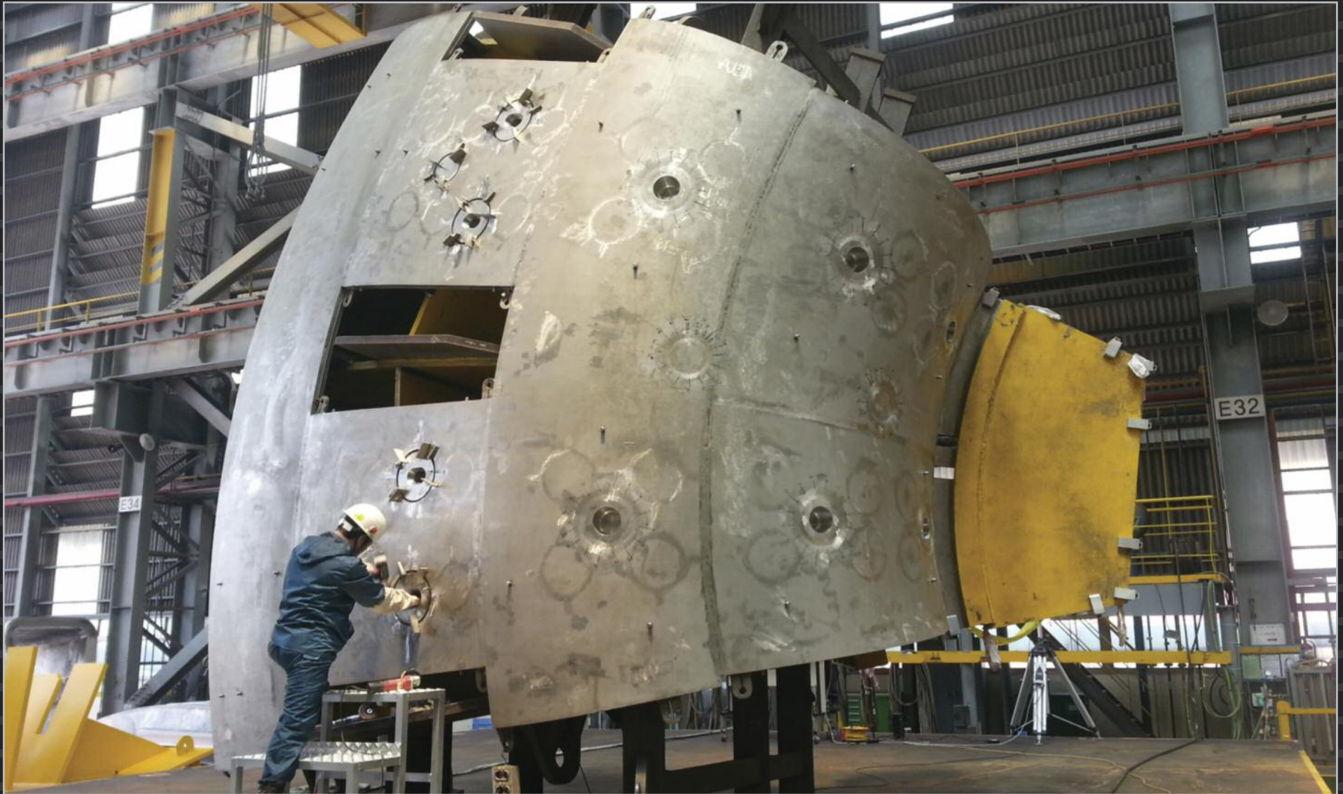
Manufacturing of the ITER vacuum vessel is underway in Korea, which is responsible for procuring two sectors out of nine. Pictured: welding operations at Hyundai Heavy Industries in Ulsan on an inner shell upper section – only a small part of one sector.
