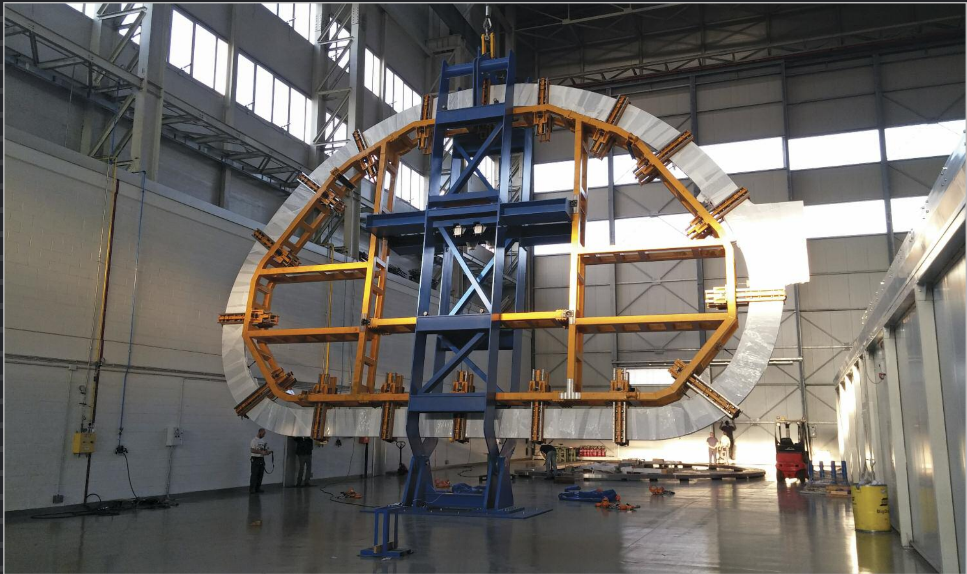
Inside of the large D-shaped toroidal field winding packs, specially grooved stainless steel radial plates, plus covers, will hold the conductor in place. In Europe, manufacturing is underway on seventy 13 x 9 m radial plates.
