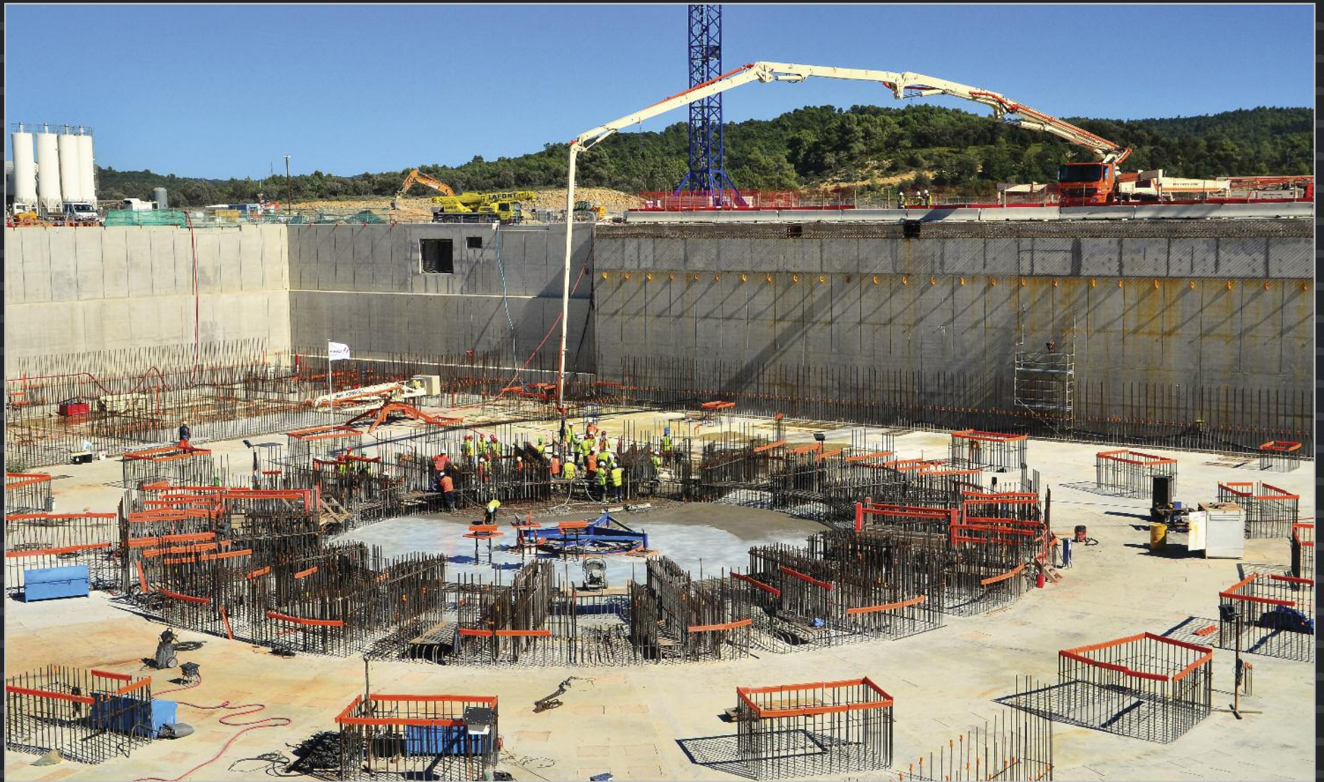
Four years of work in the Tokamak Pit to create the ground support structure and foundations of the Tokamak Complex are brought to a successful conclusion as the last segment of the B2 slab – the basemat that will support the machine and systems – is poured. August 2014
