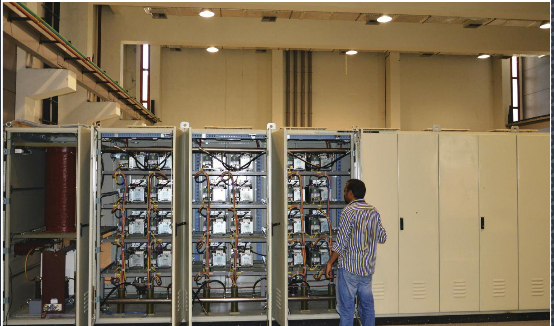
At ITER India, the high voltage power supply for ion cyclotron radio frequency heating (ICRH) is readied for testing.
