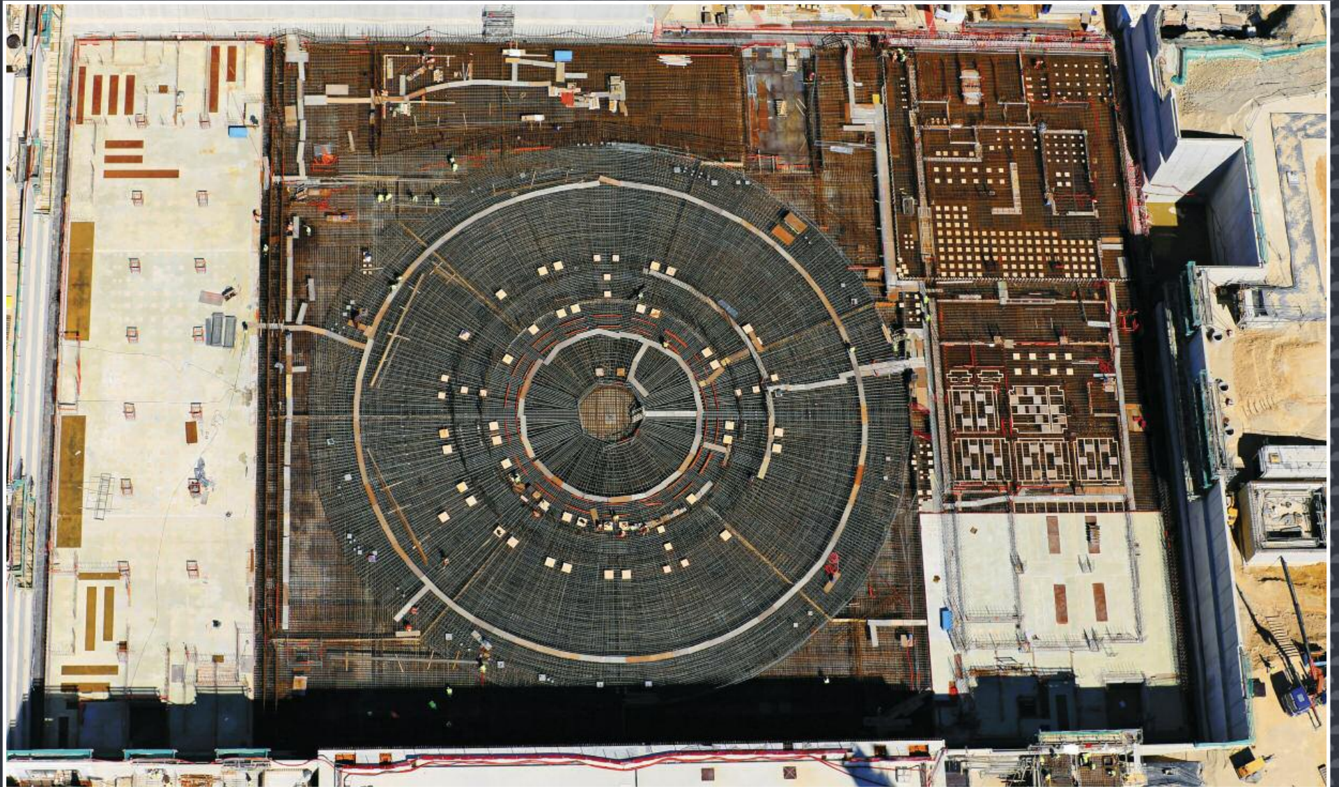
The Tokamak Complex is a suite of three buildings on a common foundation. On the left, the finished basemat slab of the Diagnostics Building. On the right, pouring is underway on the Tritium Building slab. In the central area, the circular pattern of rebar that will support the machine. April 2014
