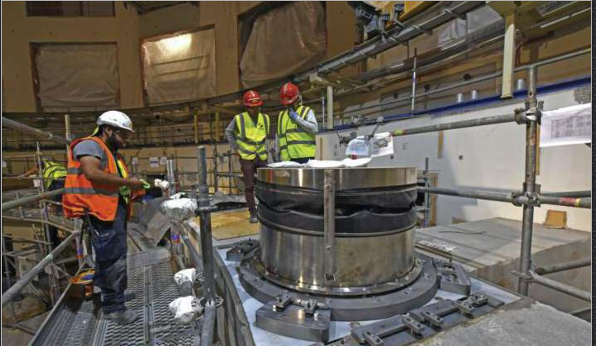
Each of the 18 cryostat bearings rests on a steel transition piece that is half embedded in the concrete crown. A high-strength top plate (3.5 tonnes of steel) is positioned on the transition piece to receive the bearings with a mechanical blocking mechanism worthy of a Swiss watch. September 2019
