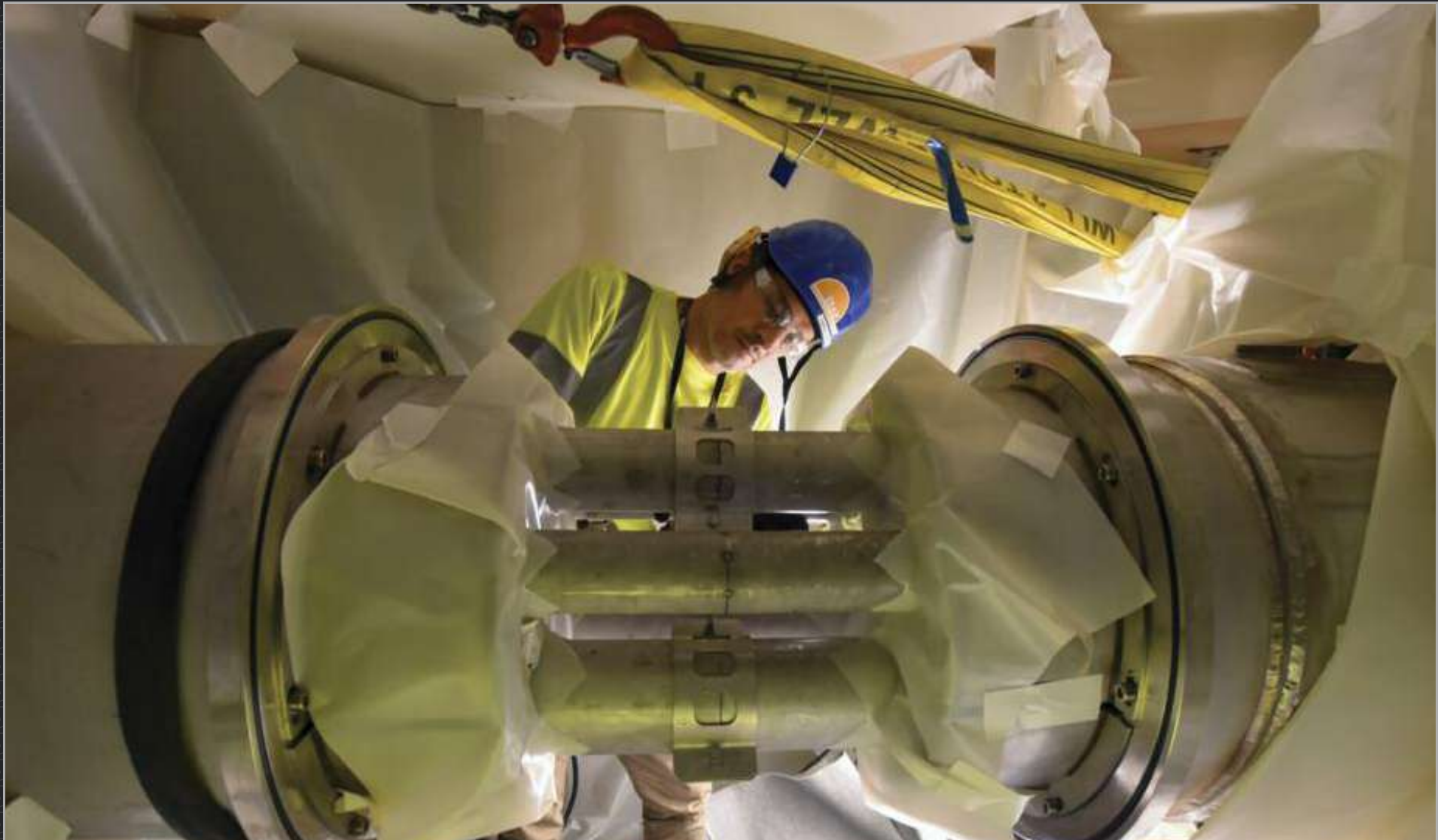
Cooling fluids produced in the cryoplant are delivered to the machine through high-technology cryolines developed by India. Looking from the outside like ordinary steel pipes, each section can host up to seven individually insulated lines. October 2019
