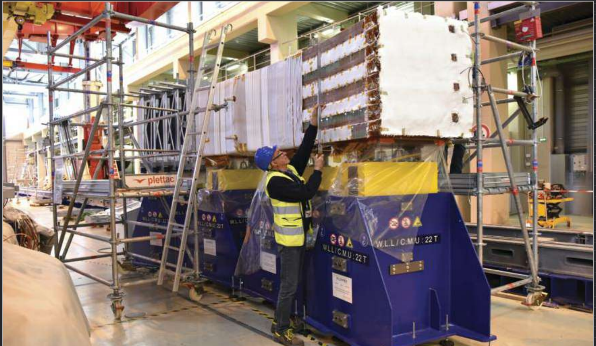
This segment of mockup coil faithfully mimics poloidal field coil #5 (PF5) and its eight stacked double pancakes. It is used in 2019 to test winding pack impregnation, before the operation is carried out on the production coil. March 2019
