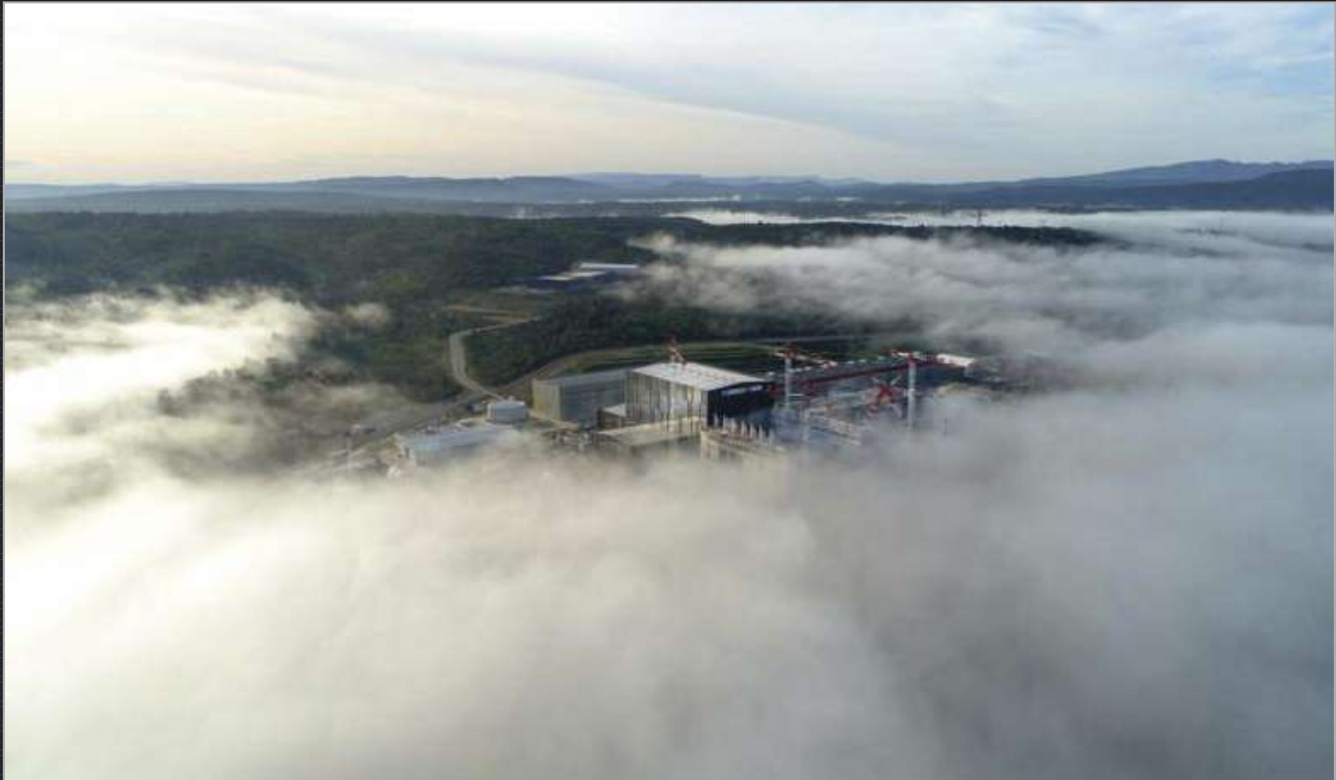
Early one autumn morning, mist from the Durance River partially obscures the construction site. ITER is nestled in the hills of Provence, about one hour north of Marseille. October 2019
