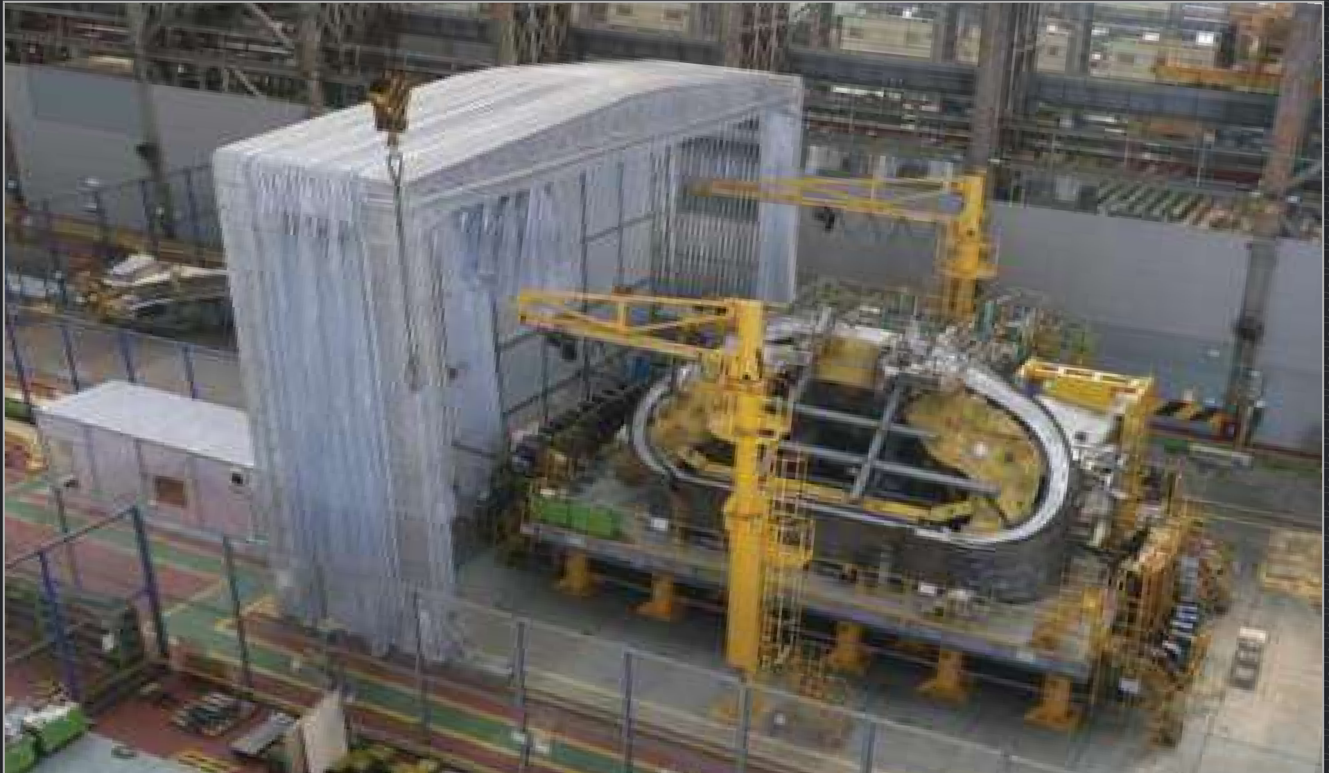
The final activities on vacuum vessel Sector #6 are underway now at Hyundai Heavy Industries, as four completed segments (plus upper and lower port stub extensions) are assembled into the final D-shaped component. Korea is procuring four of ITER's nine vacuum vessel sectors.
