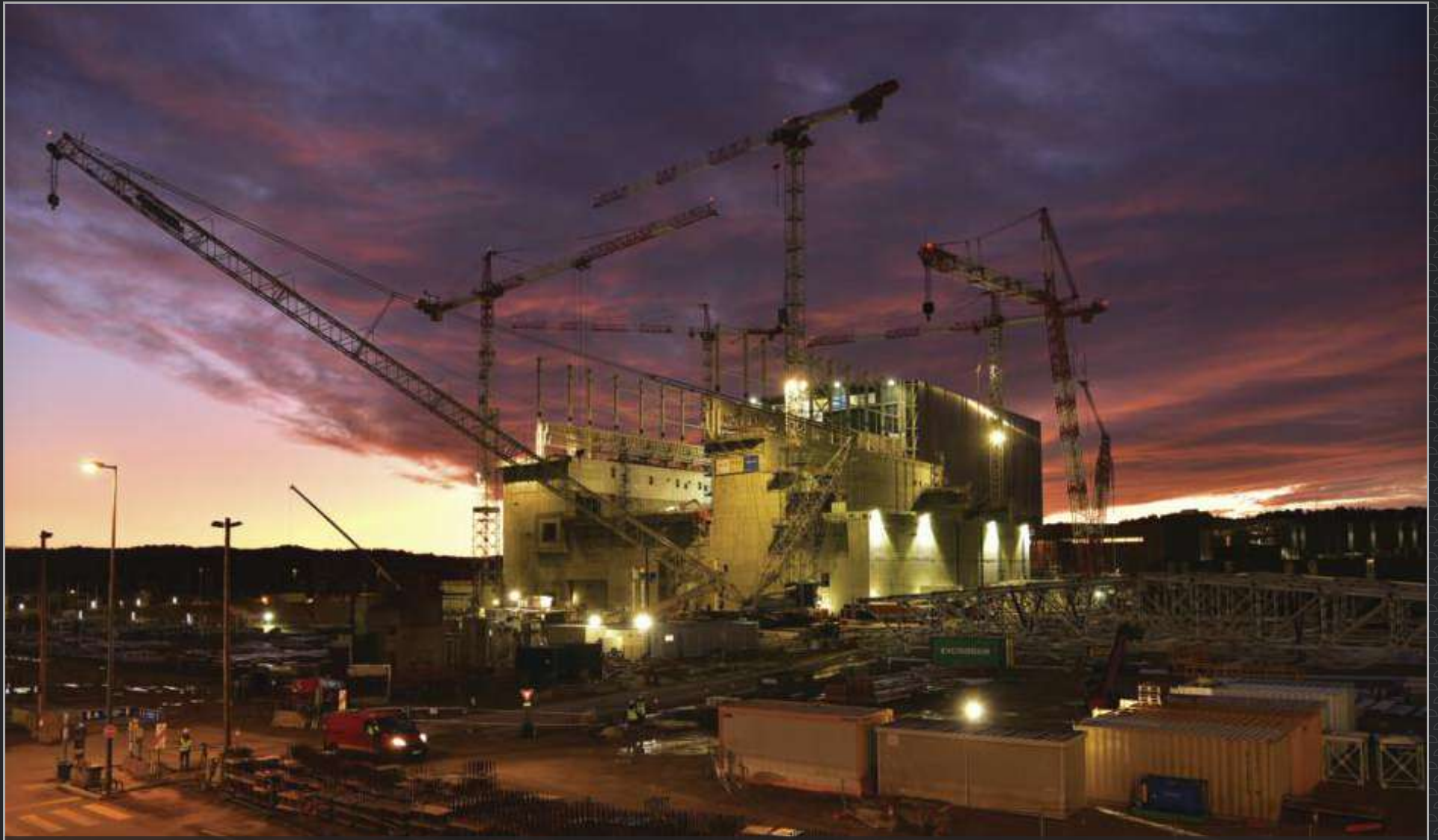
Over nine days in December, five pre-assembled modules for the roof of the crane hall are lifted into place. The first operation takes place very early in the morning. December 2019
