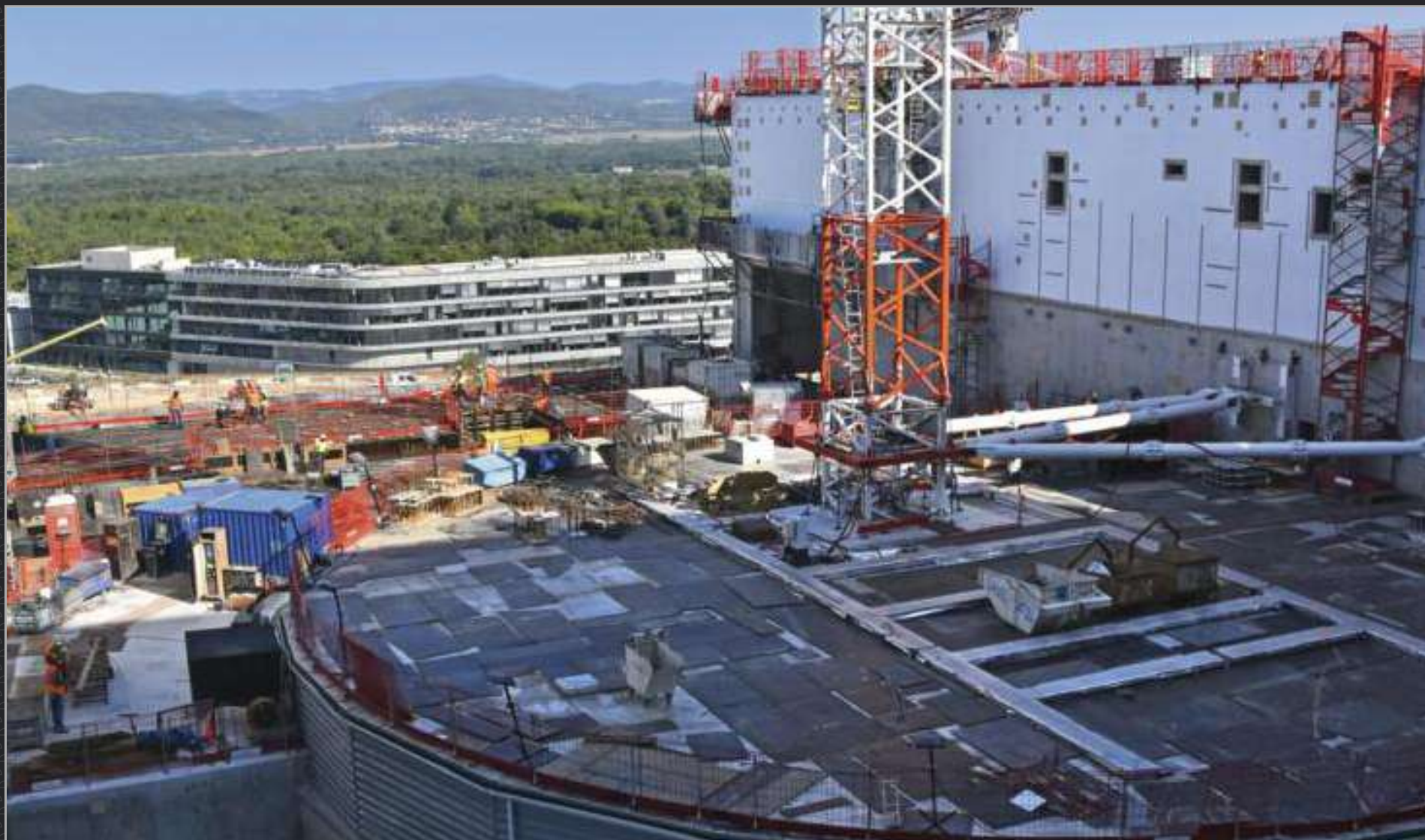
On 7 November, Fusion for Energy, the European Domestic Agency, and its contractors carry out the last concrete pour for the Tokamak Building. In all, six million work hours, performed by 850 people, were required for this project “of unusual technical complexity,” according to consortium leader Vinci Construction. November 2019
