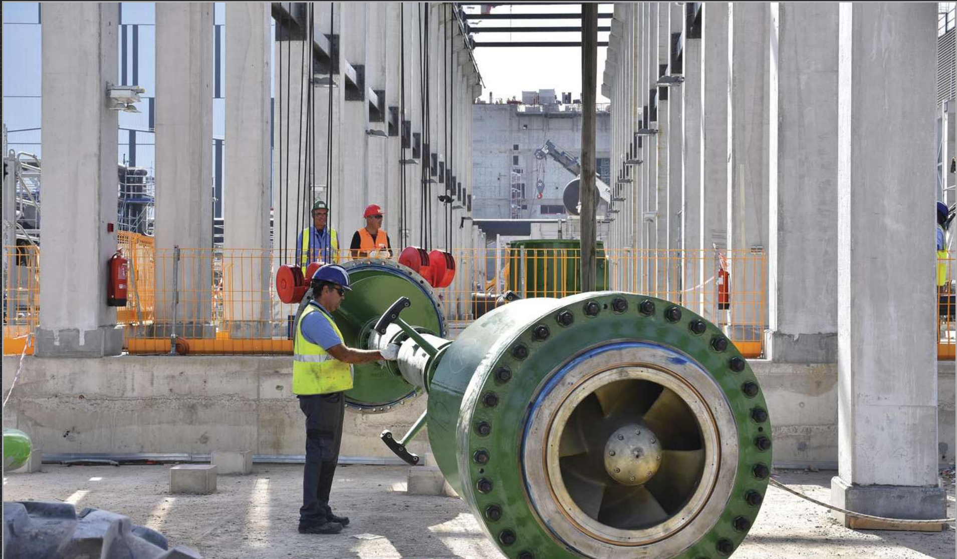
As part of the heat rejection process, 13 vertical turbine pumps will take cooling water from deep in the hot basins and circulate it to the cold basin through the heat exchangers. The six-tonne vertical shafts (pictured) must be perfectly positioned and balanced to withstand the force of the water and the rotating impellers. September 2019
