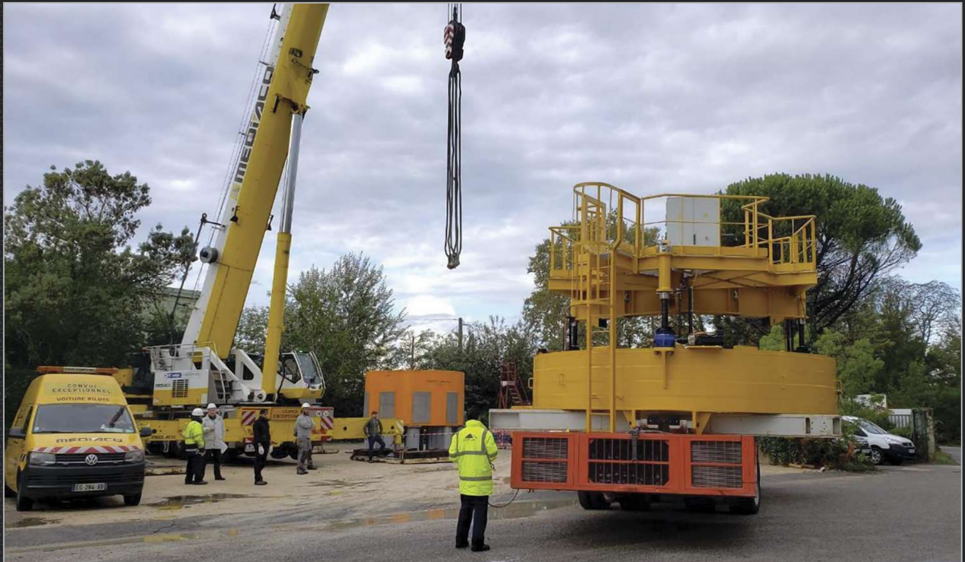
Factory acceptance testing of the central solenoid module lifting fixture is underway in Bouc Bel Air, France. The 18-metre-tall electromagnet will be assembled in the ITER Assembly Hall using tooling supplied by US ITER.
