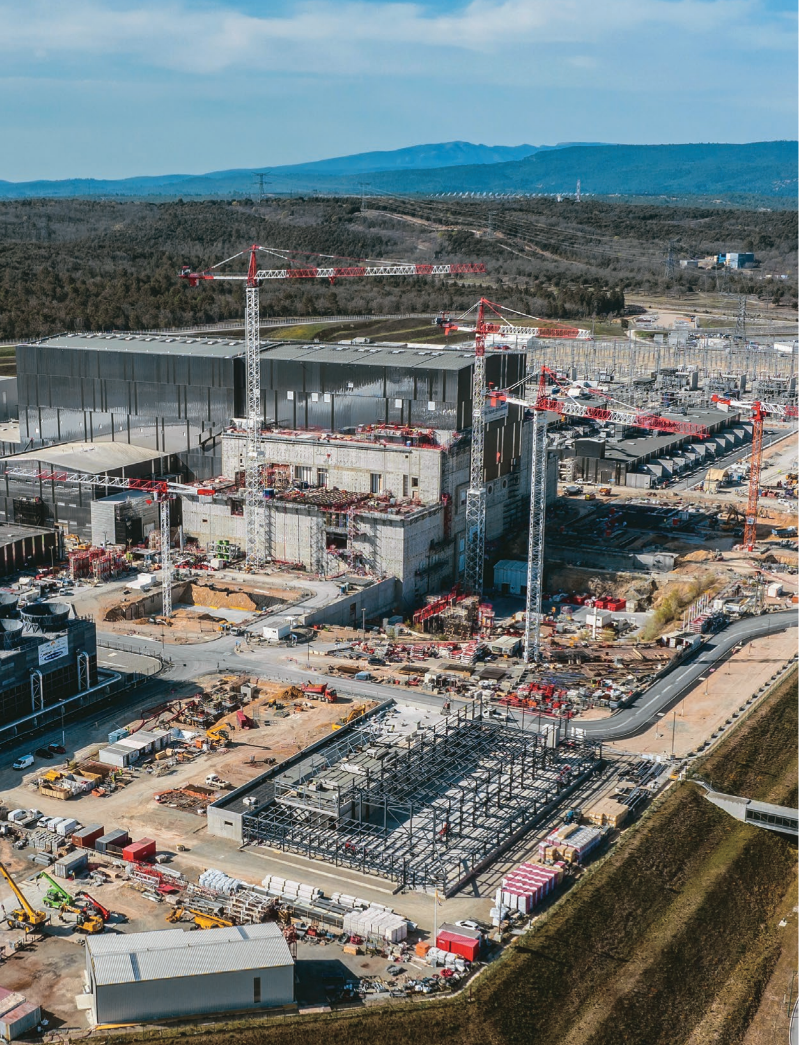
Visible progress on the worksite in 2022: the Tritium Building (concrete, centre) and the Control Building (foreground).
