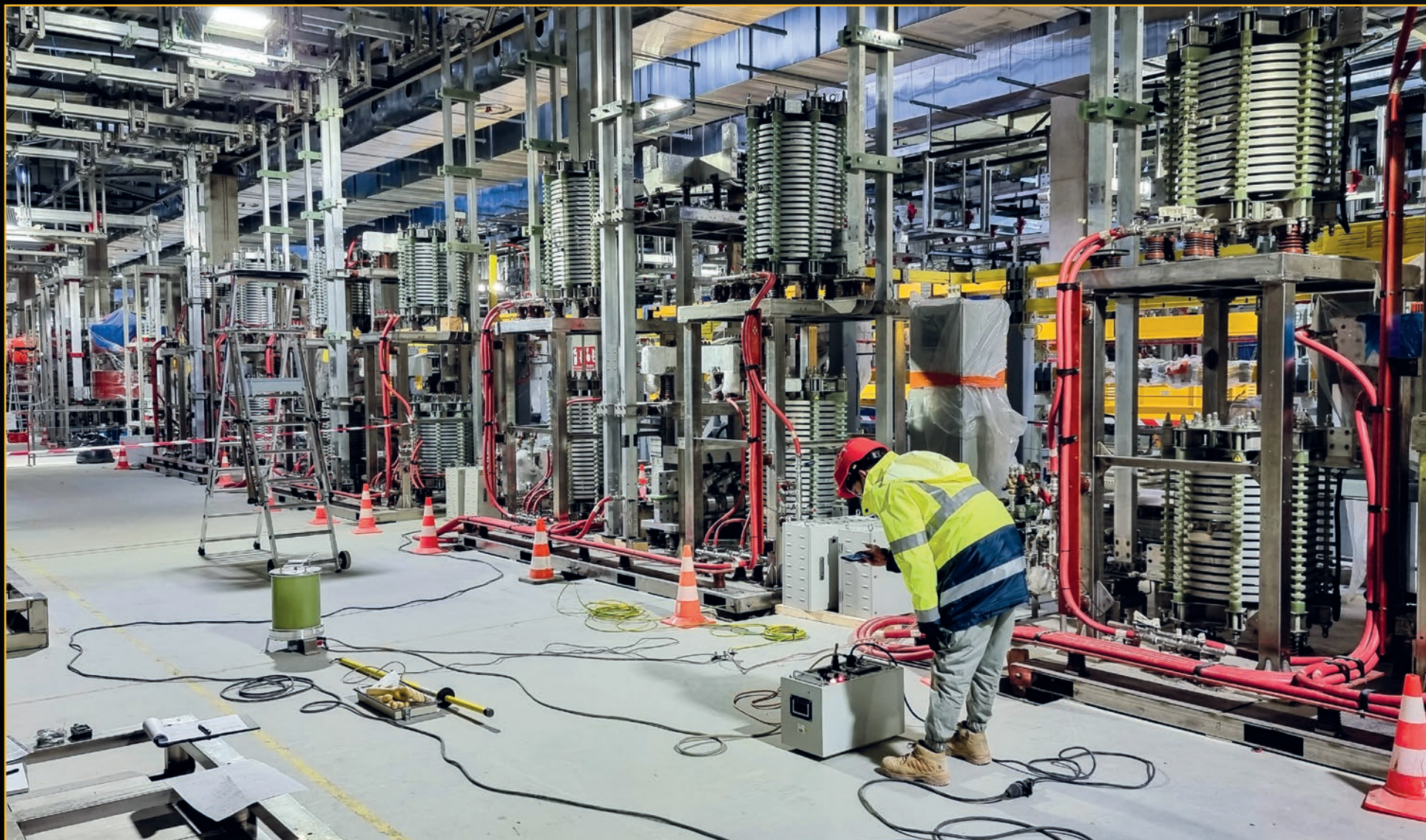
The installation of Korean-made AC/DC converters (17 units) in the Magnet Power Conversion buildings is progressing. This photo shows the insulation voltage test of the AC/DC converters that will provide current to the correction coils.
