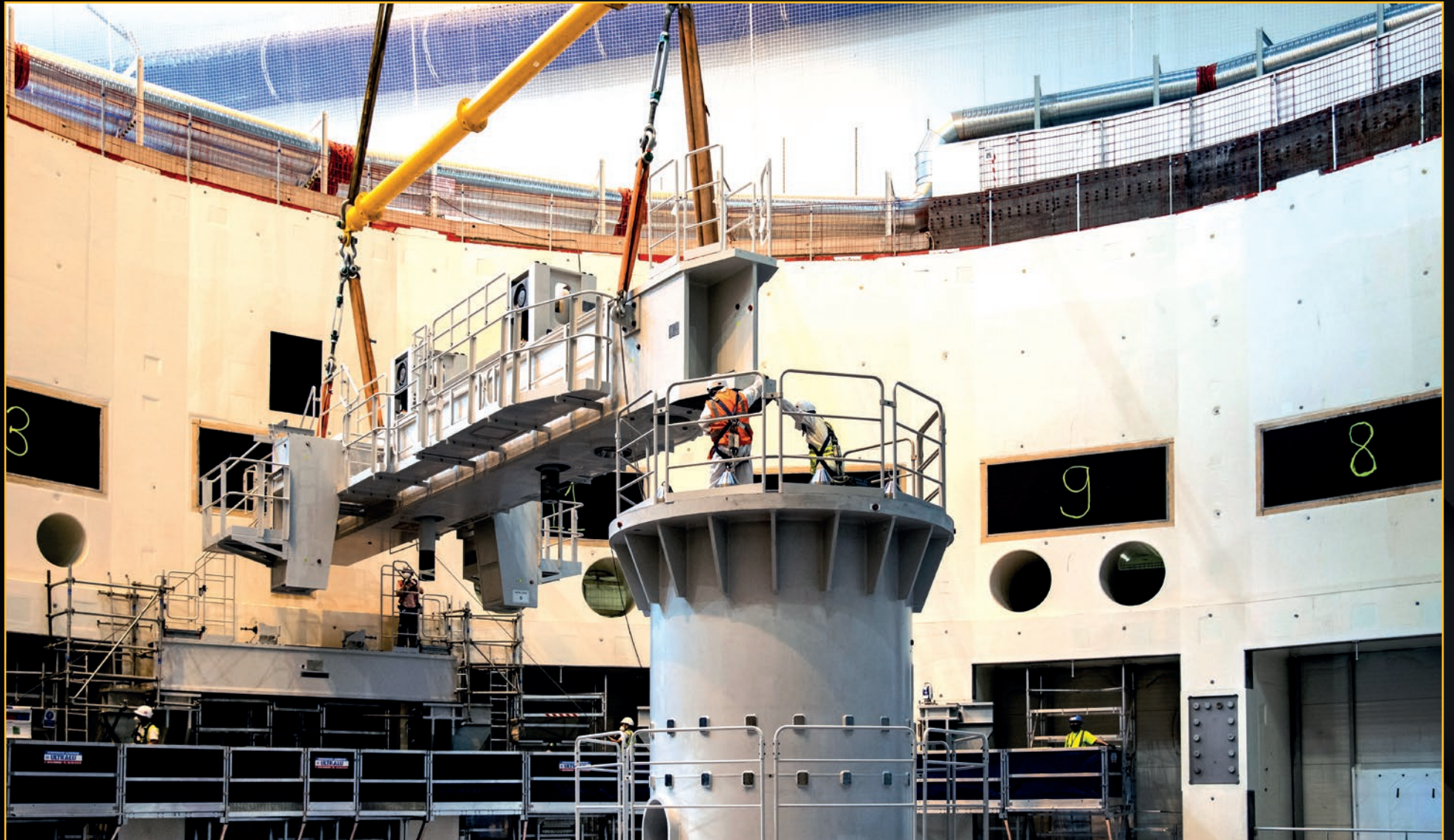
Nine radial beams docked between the central column and brackets on the wall will support the sections of the vacuum vessel as they are welded in the pit. Precise positioning is critical to the alignment of the machine torus. September 2021
