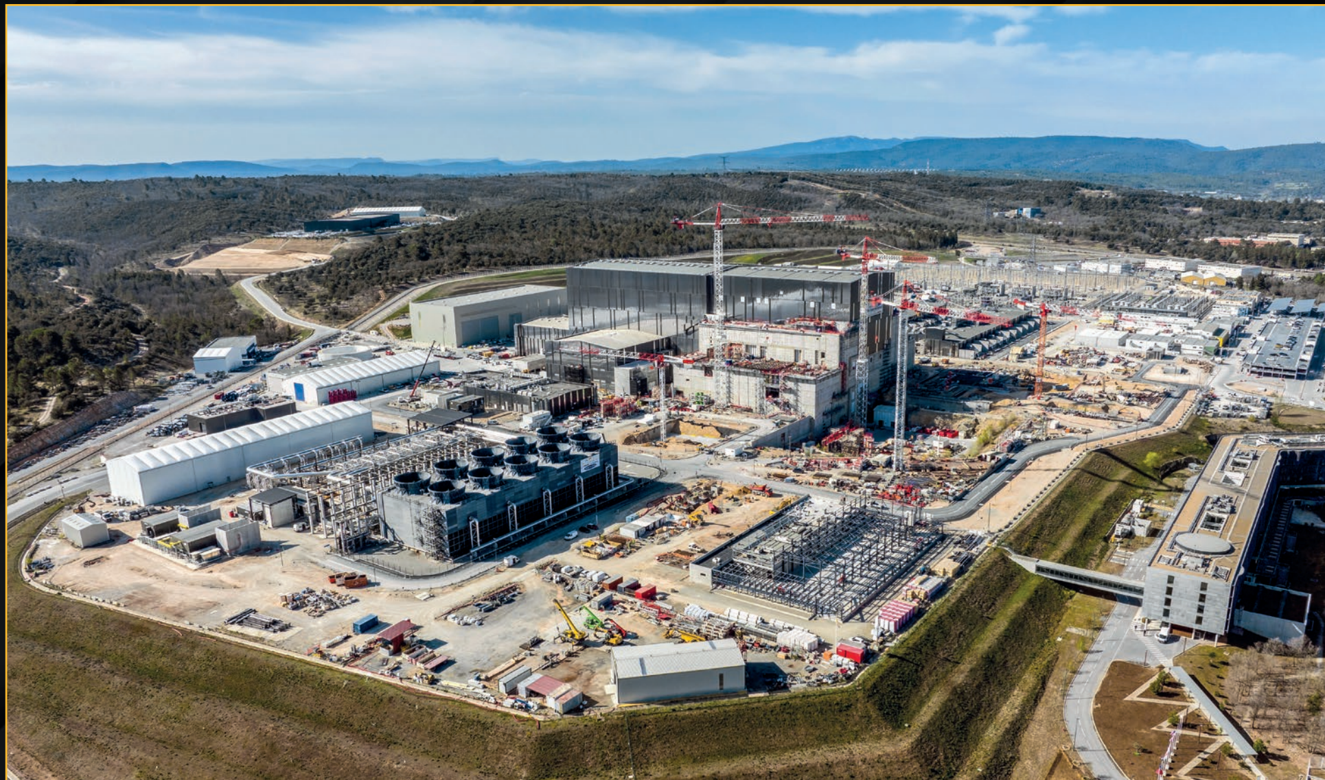
Around the central Tokamak Complex are all of the industrial plant systems—cooling, power, cryogenics, heating, fuel cycle, diagnostics—that enable the operation of the ITER machine. April 2022
