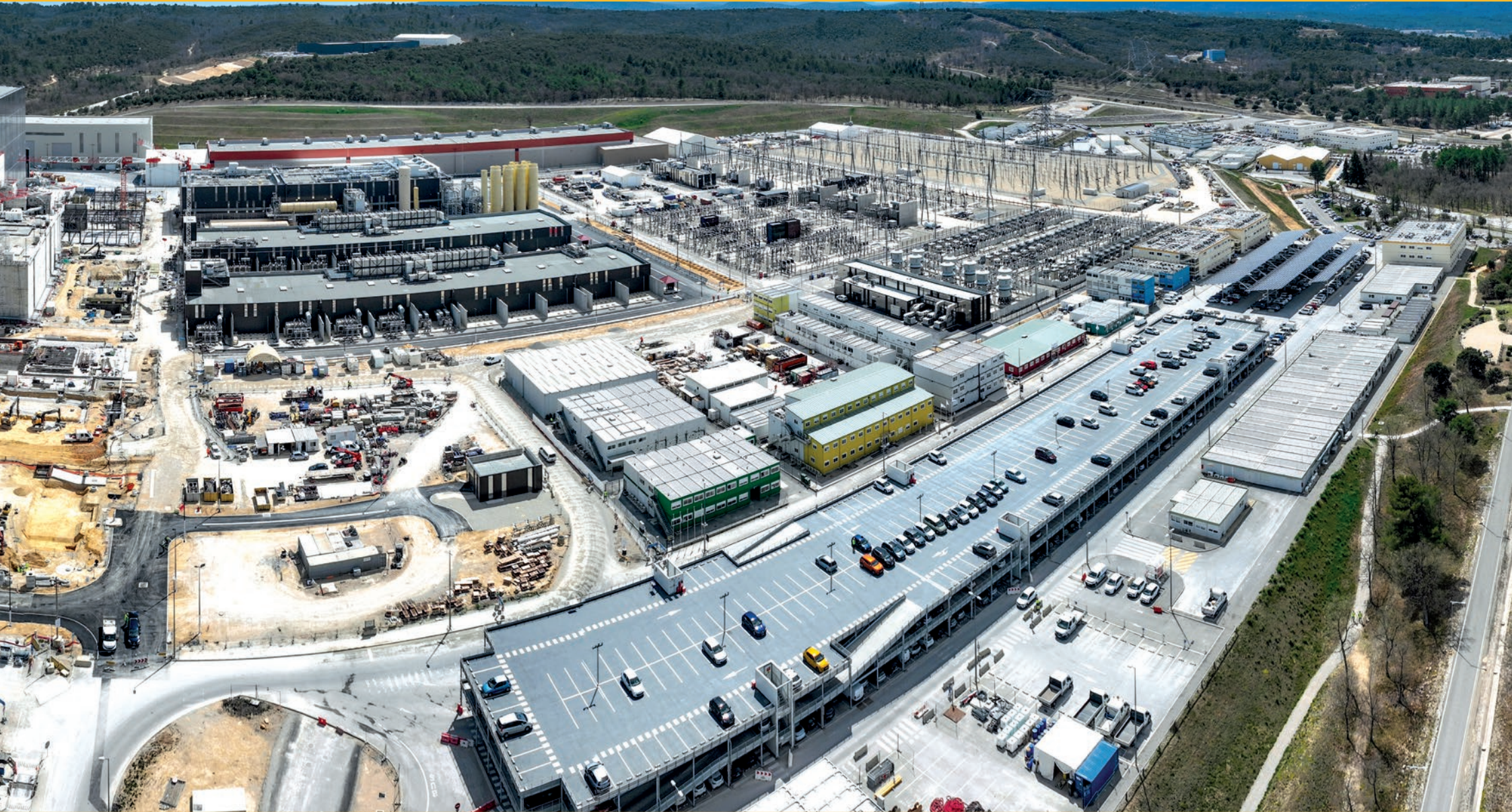
The ITER scientific installation is rising on this rural site in southern France. Eighty-five percent of the infrastructure required for First Plasma is now in place. April 2022
