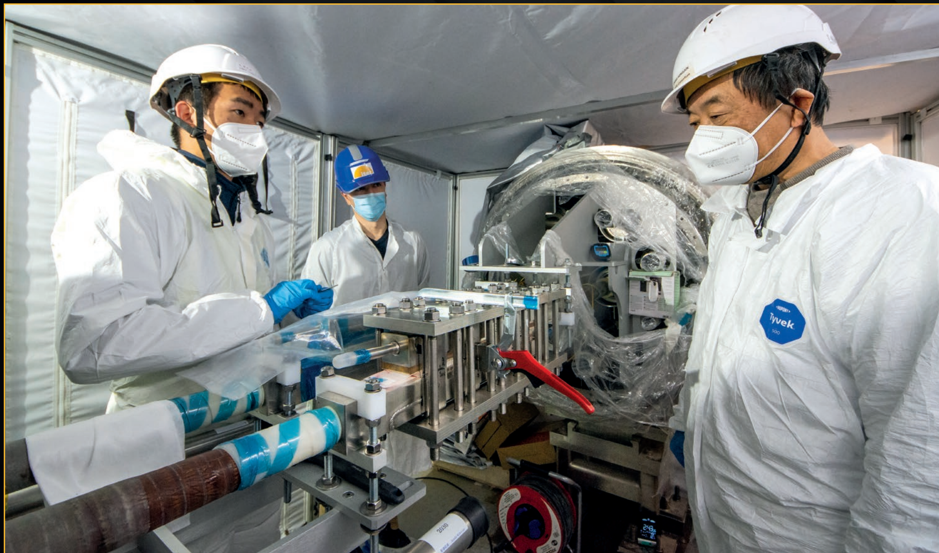
Tokamak assembly is a mix of spectacular operations, such as when giant components are lifted and positioned with complete accuracy, and less visible activities requiring near surgical-like precision. Creating the superconducting joints that join magnet feeder segments (photo) falls into the latter category. March 2022
