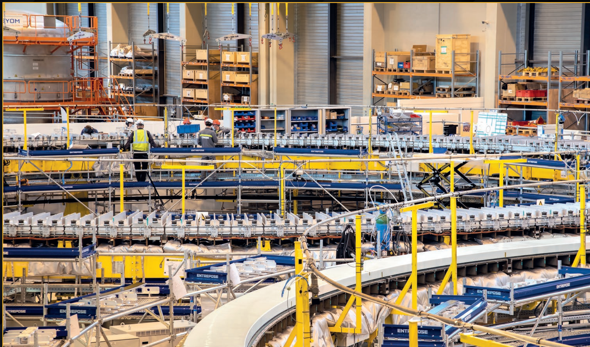
In its on-site winding facility, the European Domestic Agency Fusion for Energy (F4E) is producing four poloidal field coils. Each one is formed by stacking layers of conductor called double pancakes, pictured here in production. January 2021
