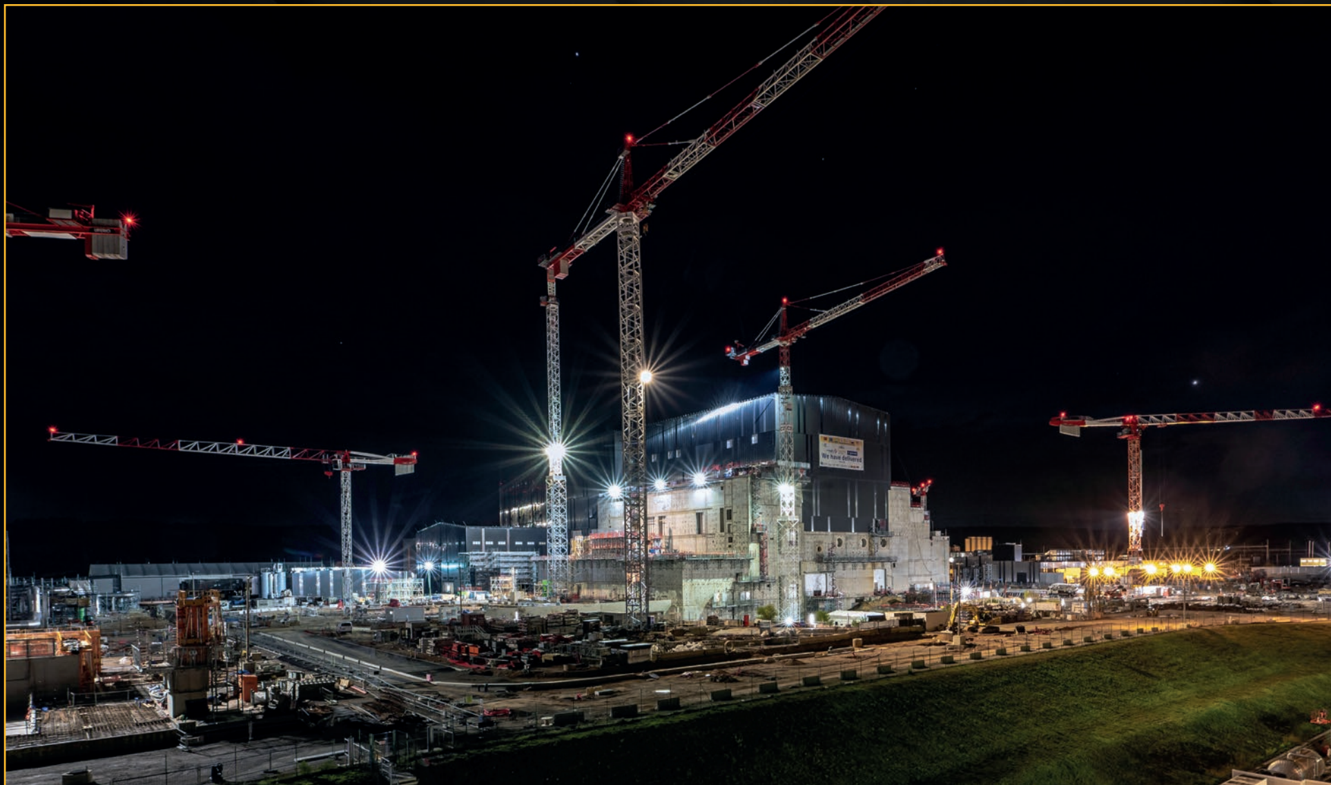
Work continues into the night on the ITER site. Inside the tall Tokamak Building, teams are assembling the ITER machine from bottom up. November 2021
