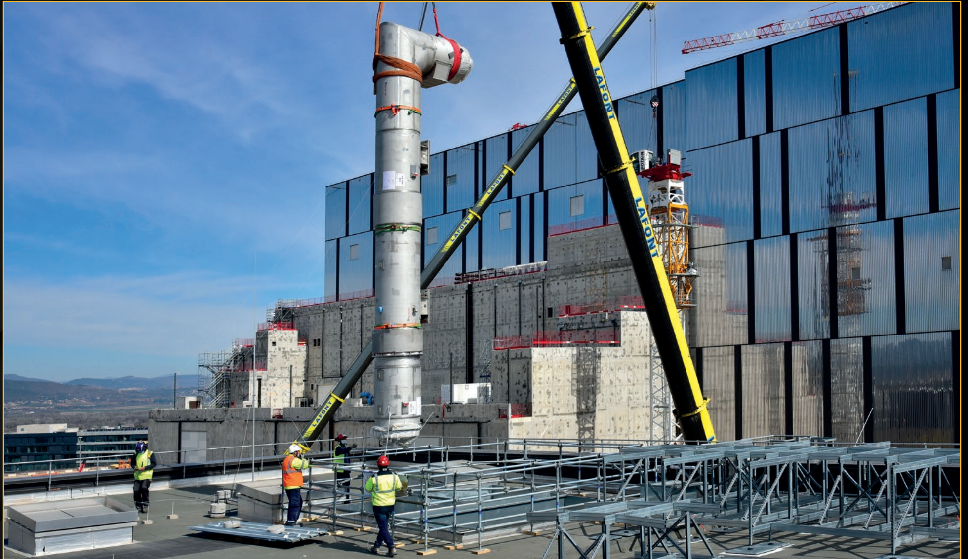
A cryoline spool is installed in the ITER cryoplat, part of the multi-process piping system that will transport cooling fluids to the Tokamak Building. March 2021
