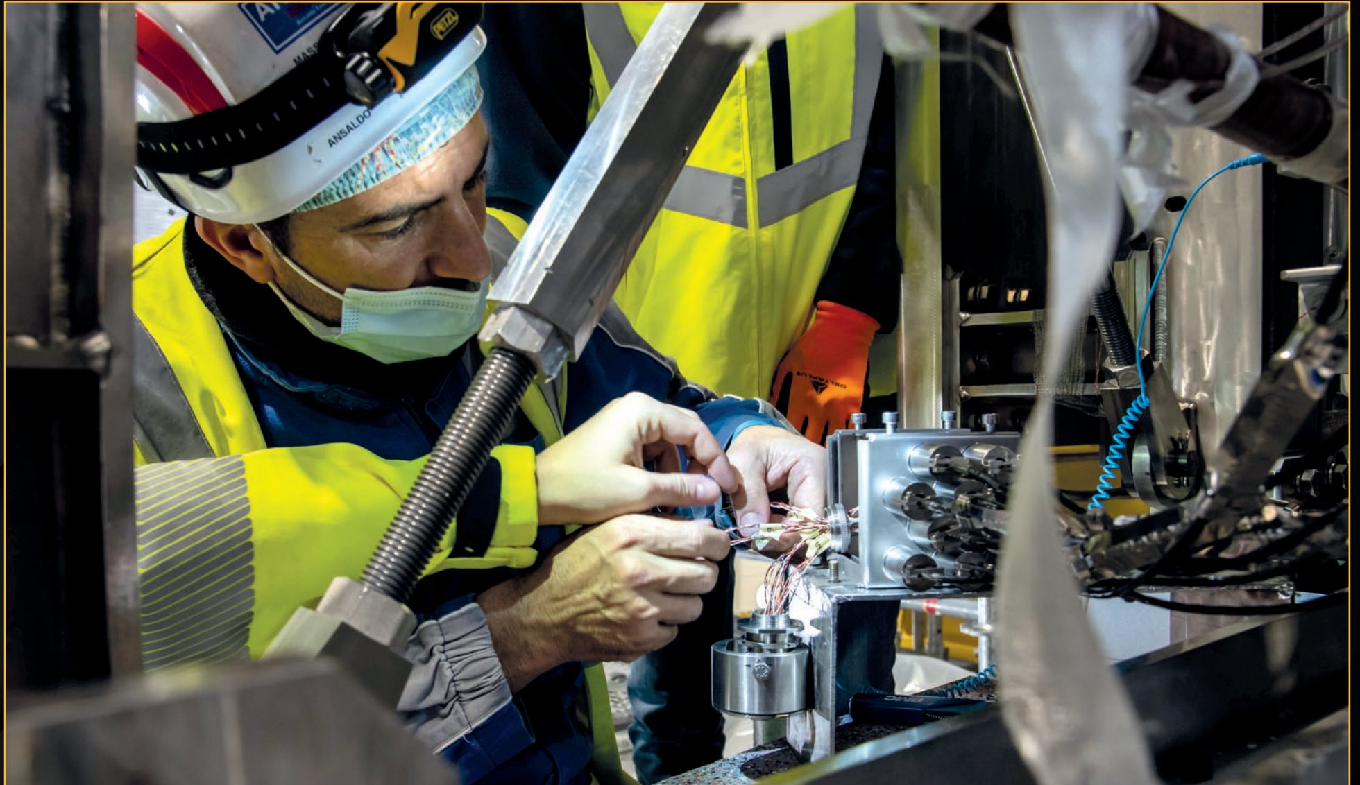
Diagnostics are added to the toroidal field coils before they are moved to assembly tooling. March 2021
