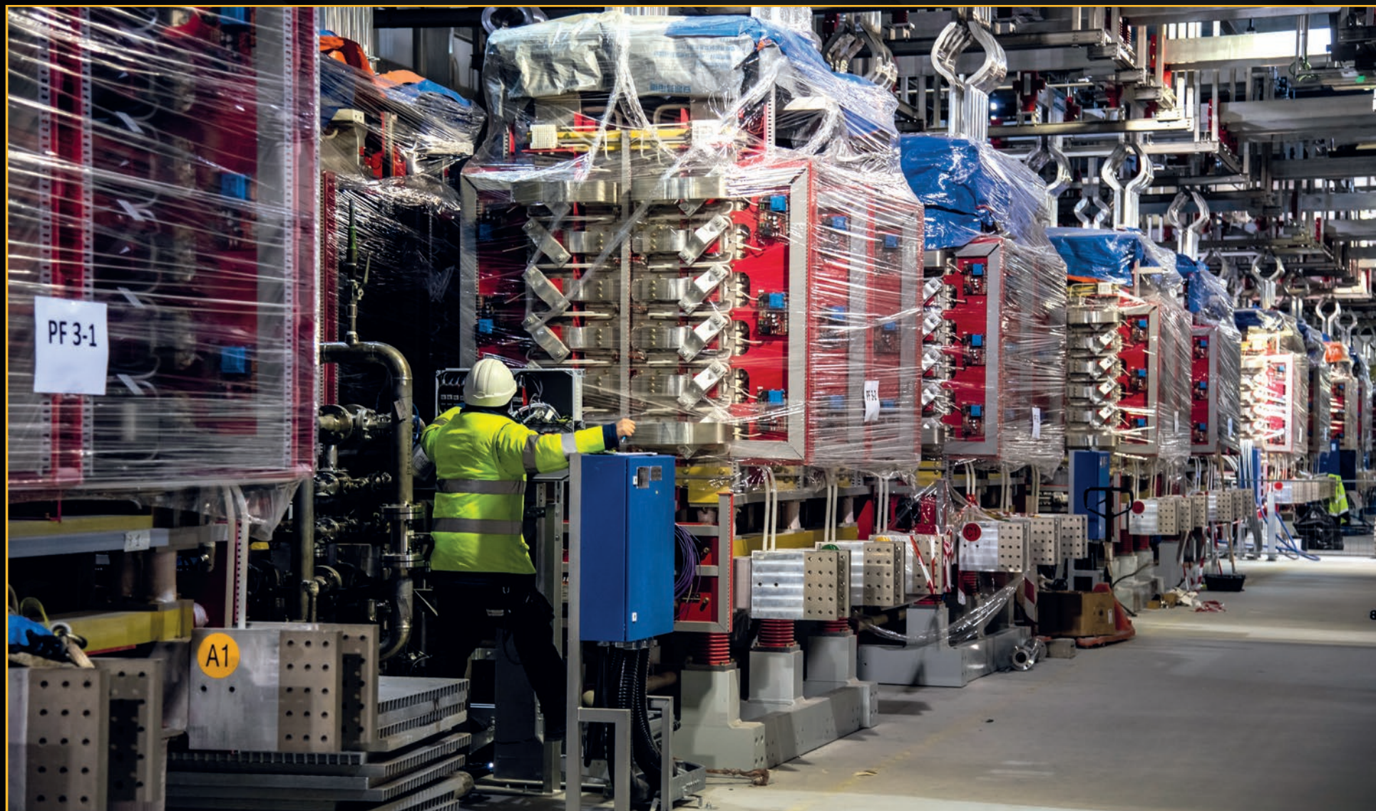
Equipment from China has been installed in the Magnet Power Conversion buildings, which are the «stepping stones» between the power arriving at the ITER switchyard at 400 kV and the voltages required by the ITER magnets. In particular, China has supplied the 14 AC/DC converters that will provide controllable current/voltage to ITER's six poloidal field coils.
