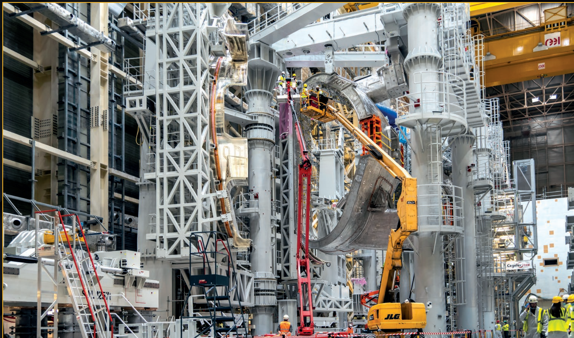
On these twin sector sub-assembly tools in the Assembly Hall, a vacuum vessel sector can be associated with its thermal shield and two toroidal field coils to form a sector module, or one-ninth of the ITER plasma chamber. One sector module was finalized in 2021 and a second is underway. January 2022
