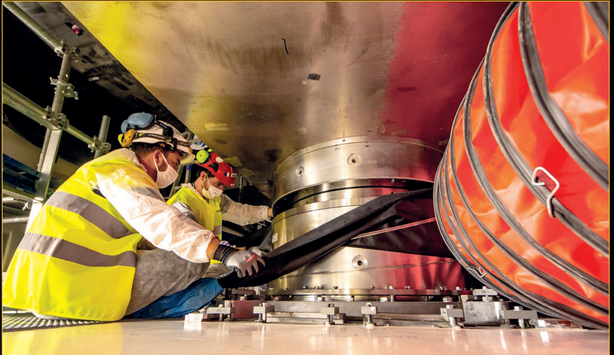
Once installed, components and materials must be kept in good condition until they enter service. Here, a worker performs a white cloth test to check for moisture on a cryostat support bearing during a preservation inspection. September 2021
