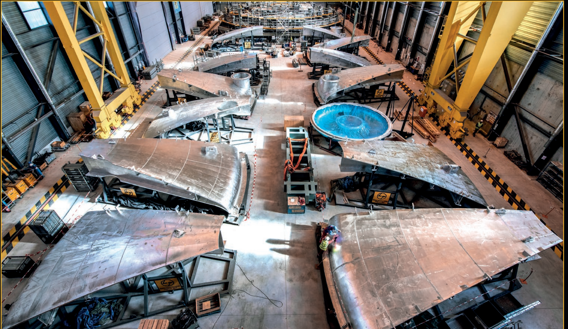
The segments of the cryostat lid arrive early in the year from India. They will be aligned and welded on the platform at the far end of the Cryostat Workshop. February 2021
