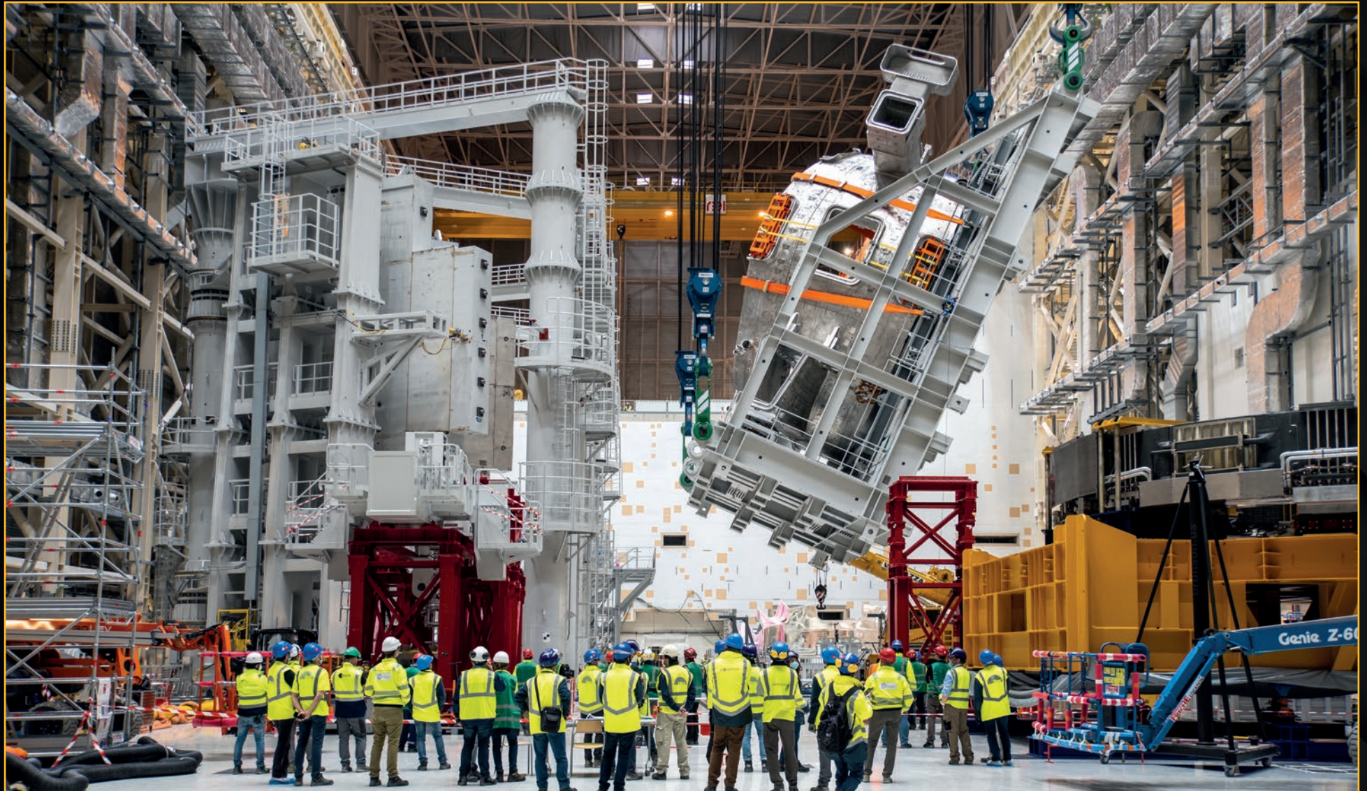
The first vacuum vessel sector to arrive at ITER—sector #6 from Korea—is upended on specialized tooling in March. In this vertical position, it can be installed on sector sub-assembly tooling and prepared for final transfer to the Tokamak pit. March 2021
