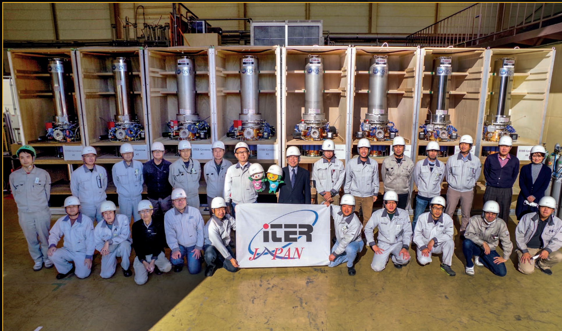
QST has procured eight gyrotrons for ITER's electron cyclotron external heating system. Four of these high technology "wave factories" have passed factory acceptance tests and will be delivered for First Plasma.
