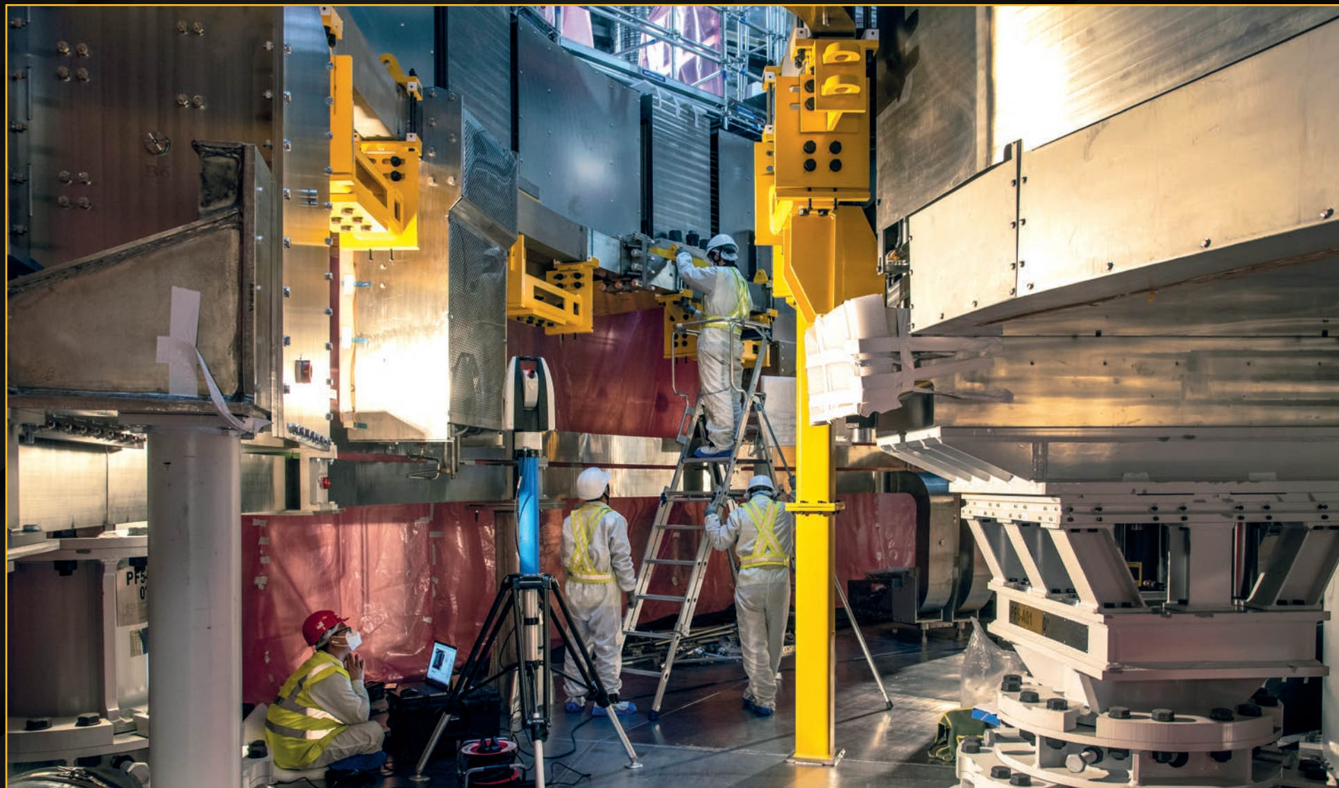
At the very bottom of the Tokamak pit, inside the “soupbowl-like” depression in the cryostat base, teams are installing captive components like the slim magnet feeder lines that will deliver cryogenic fluids and electricity to the lower poloidal field coils. March 2021
