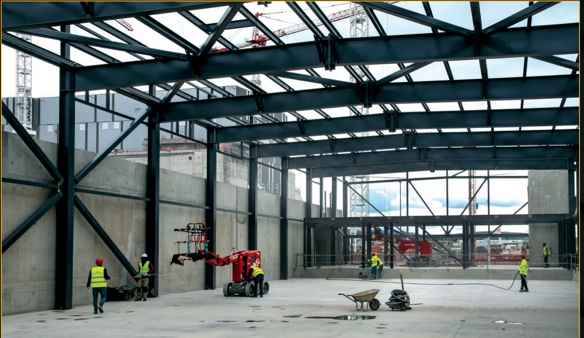
Work is advancing on the ITER Control Building. This 18 m x 43 m space will be the main control room, where scientists, engineers and operators monitor machine operation and analyze the data they receive from each pulse. May 2022
