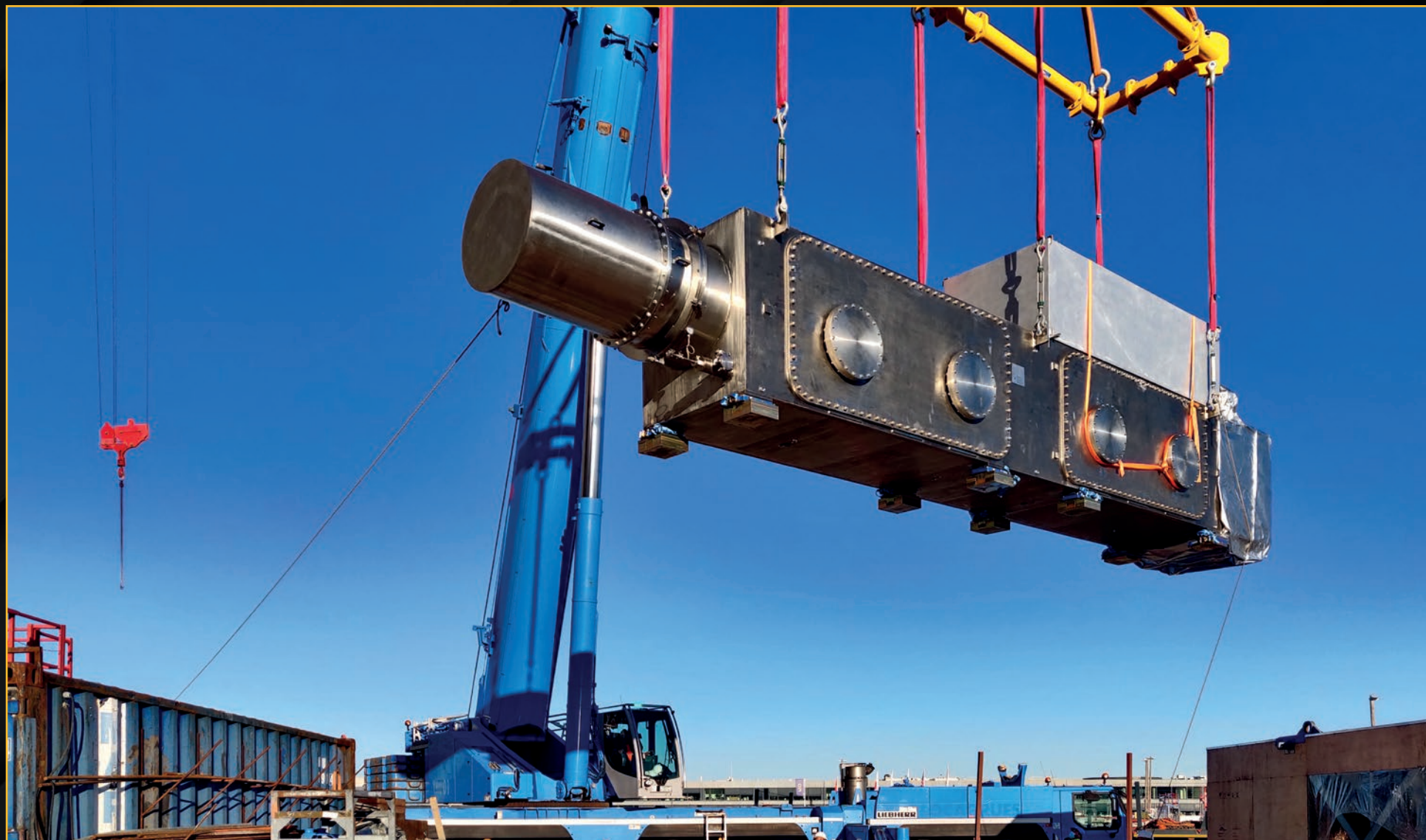
Each of ITER's 31 magnet feeders is produced and shipped in three segments by China. That's approximately 100 feeder large components that must be installed in the Tokamak Complex. January 2021
