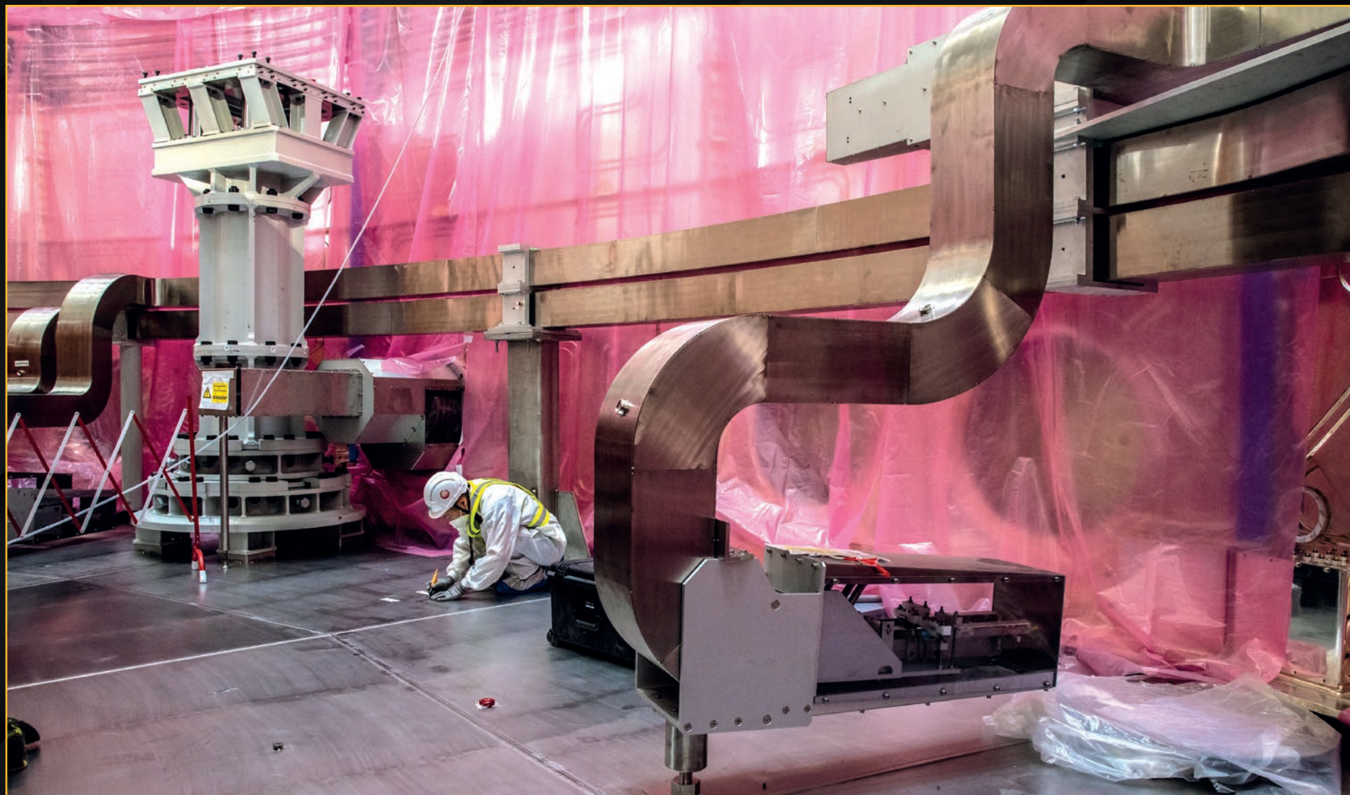
In 2021, the assembly pit is declared "ready" for the first vacuum vessel sector after all captive components (like the magnet feeders pictured here) are installed. June 2021
