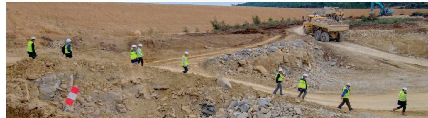
Approximately 500 construction workers were active on the ITER platform in 2011; at the peak of construction activity in 2014-2015, this number will rise to 3,000.
