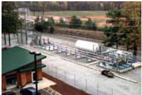
The Southwire Company facility in Carrollton, Ga., was the site of the first installation of the HTS cable. (Photo courtesy of Southwire)
