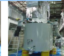
Temperature Variable Helium Refrigerator
