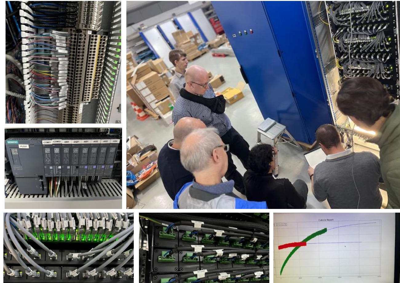
Magnetic diagnostic cubicle at Factory Acceptance Testing
