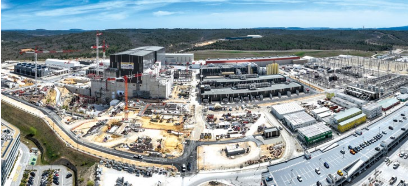
Approximately 5,000 people work on the ITER site daily, including 3,600 in construction and assembly.
