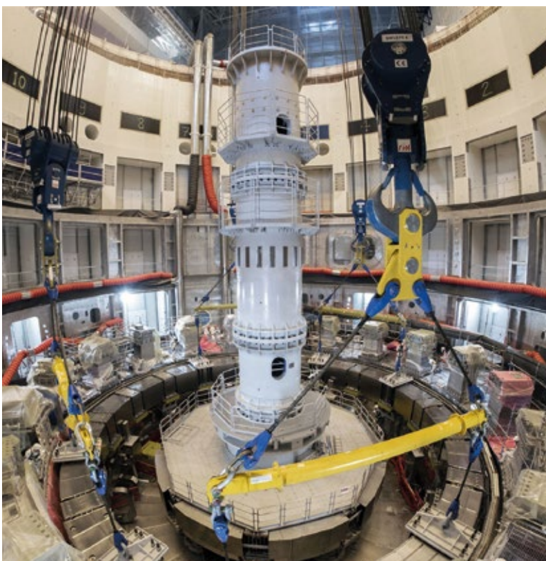
A temporary column is installed to support the vacuum vessel sectors while they are progressively installed and welded.
