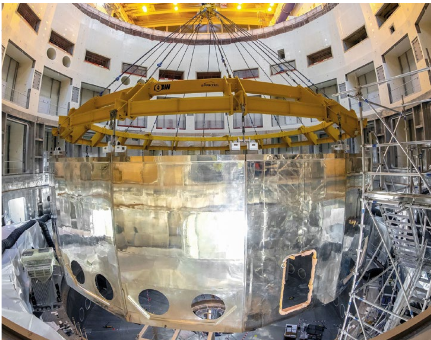
In January, the silver-plated lower cryostat thermal shield is inserted into the pit. Eighteen lift attachments facilitate the centring of the load and ensure perfect balance.
