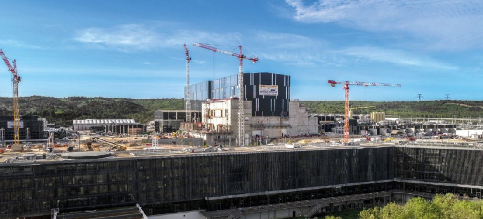
The buildings housing the ITER machine and plant are all contained on this one-kilometre-long platform, with the Tokamak Complex at its centre. Down from the platform (in the foreground), ITER Headquarters offers desks and meeting spaces for approximately 800 people.
