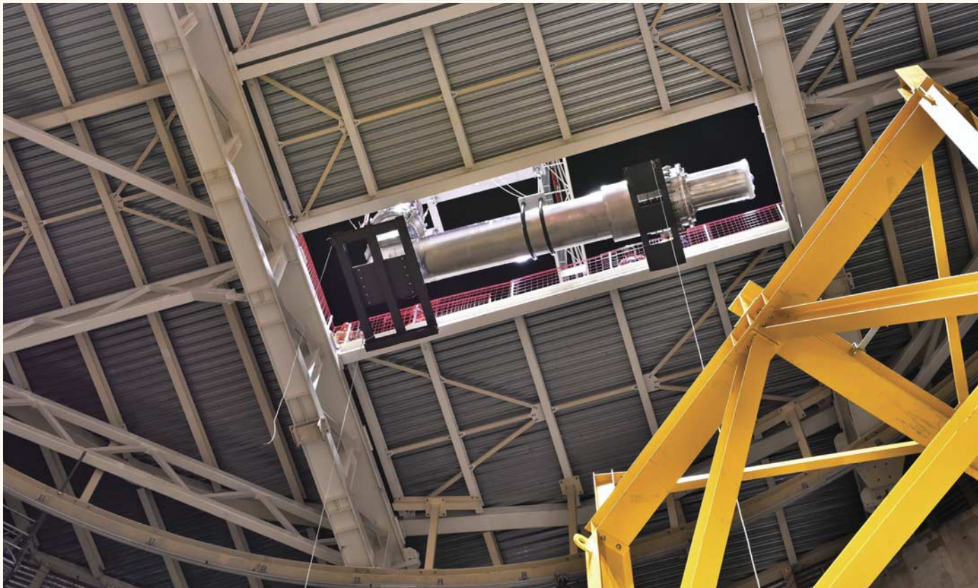
In November, the first machine component is lowered into the Tokamak Pit – a 10-metre, 6.6-tonne segment of magnet feeder delivered by China.
