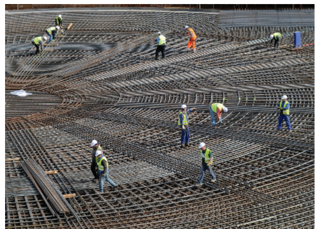
The most heavily reinforced part of the Tokamak Complex basemat is the central portion, located under the machine.
