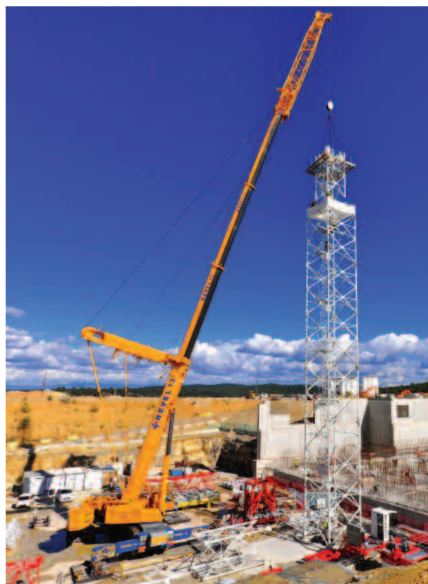
In the last months of 2014, five tall cranes are installed in and around the Tokamak Pit to prepare for the start of wall construction.
