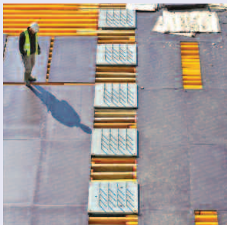
Work on the Tokamak Complex concrete slab (B2) progresses in stages: propping and formwork (pictured), followed by the installation of 4,000 tons of steel rebar.
