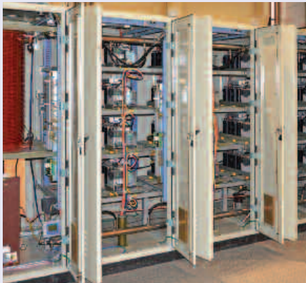
The R&D unit of high voltage ion cyclotron radio frequency power supplies is readied in India for testing.
