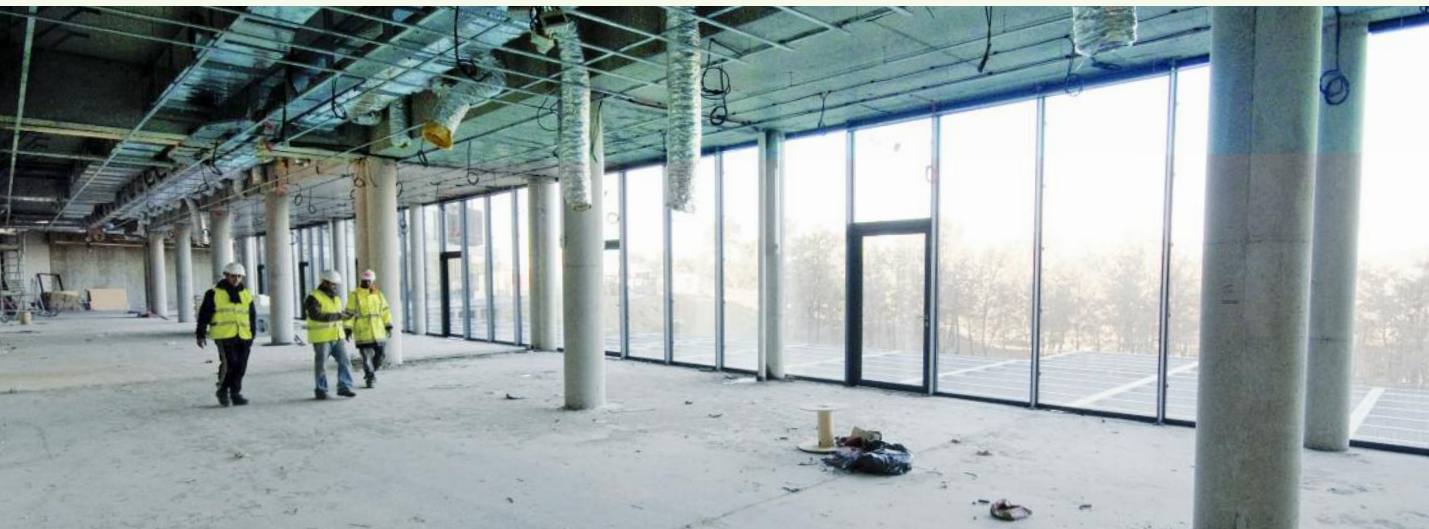
Nestled up against the northern corner of the ITER platform, the wing-shaped ITER Headquarters includes offices for 500 people, meeting rooms, a boardroom, an auditorium, a library, and a cafeteria. Photo: © F4E
