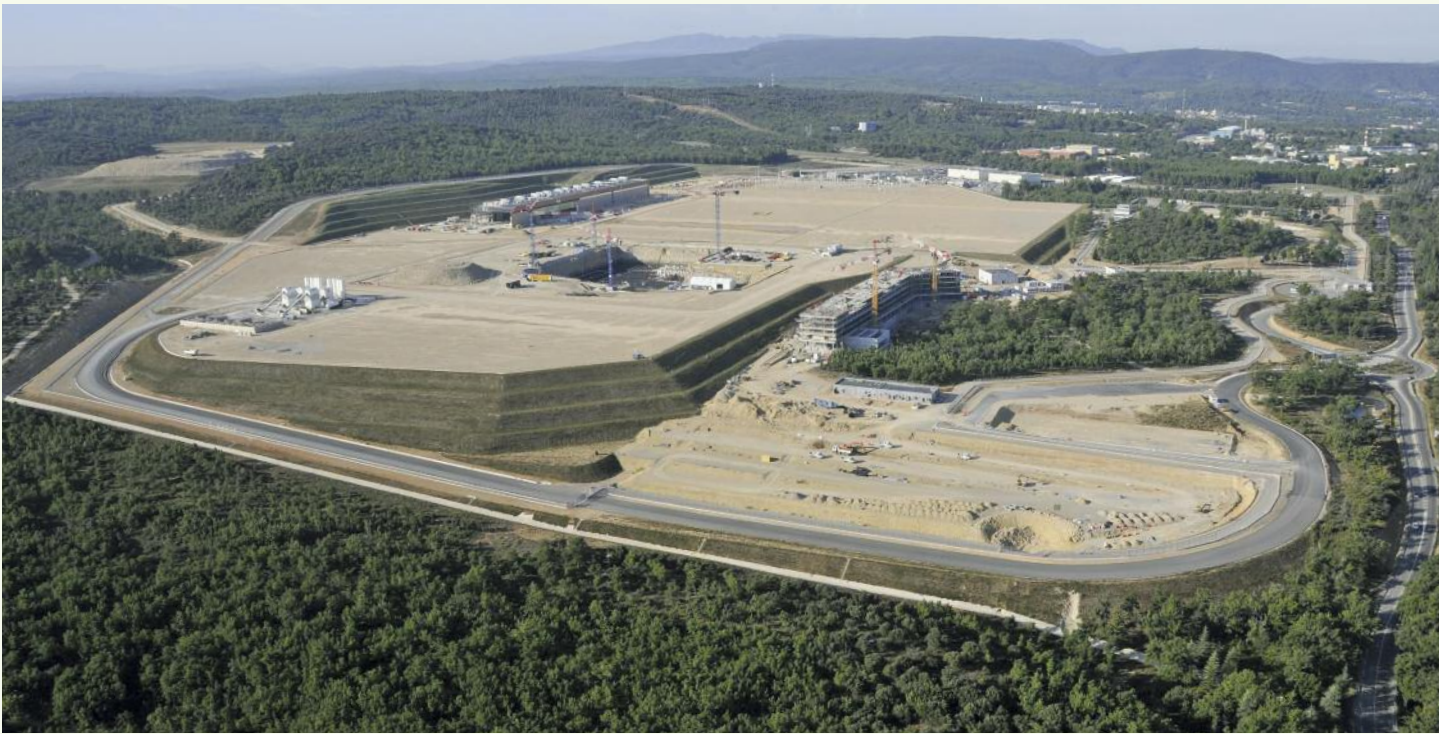
The 42-hectare ITER Platform and its surroundings in September 2011. Construction work is on-going on the Headquarters Building (right), Tokamak Seismic Pit (centre) and PF Coils Assembly building (centre-left). Photo: © Altivue-ITER Organization
