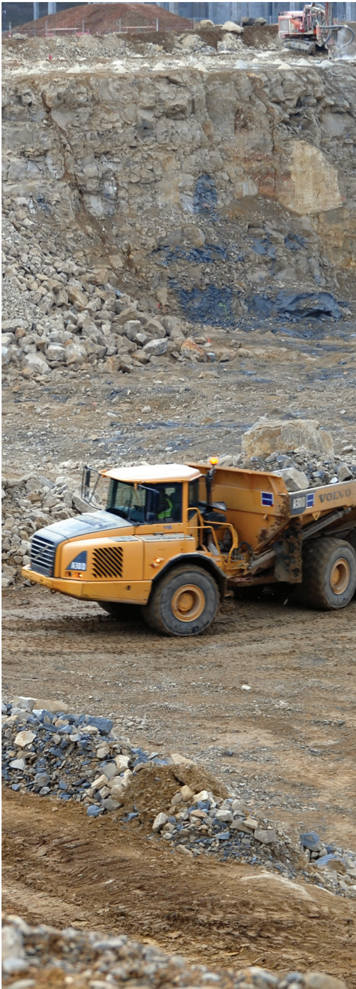
To create the Seismic Isolation Pit, home to the future ITER Tokamak Complex, diggers will excavate an estimated 210,000 cubic metres of soil and rock from the ITER platform.
