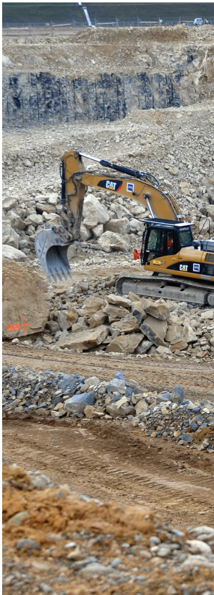
Seventeen metres deep, the Seismic Isolation Pit will house the anti-seismic foundations and retaining walls of the future Tokamak Complex.
