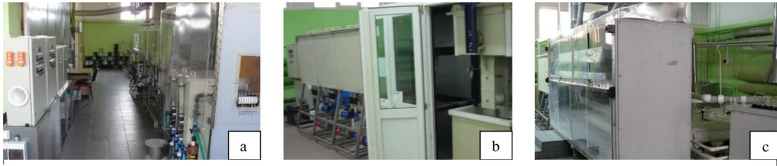
Fig. 1. The processing equipment for (a) cleaning, (b) chromium, and (c) nickel plating.
