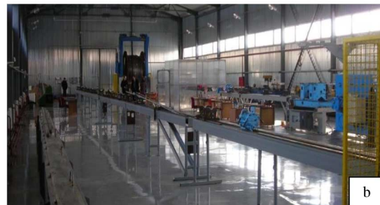
Fig. 5. Jacketing line outlook: (a) hangar and protective gallery; (b) inside of hangar.
