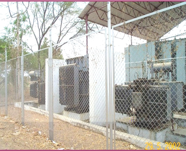
11kV (ac) Voltage Variation system: It varies input ac voltage for HV DC PS.
