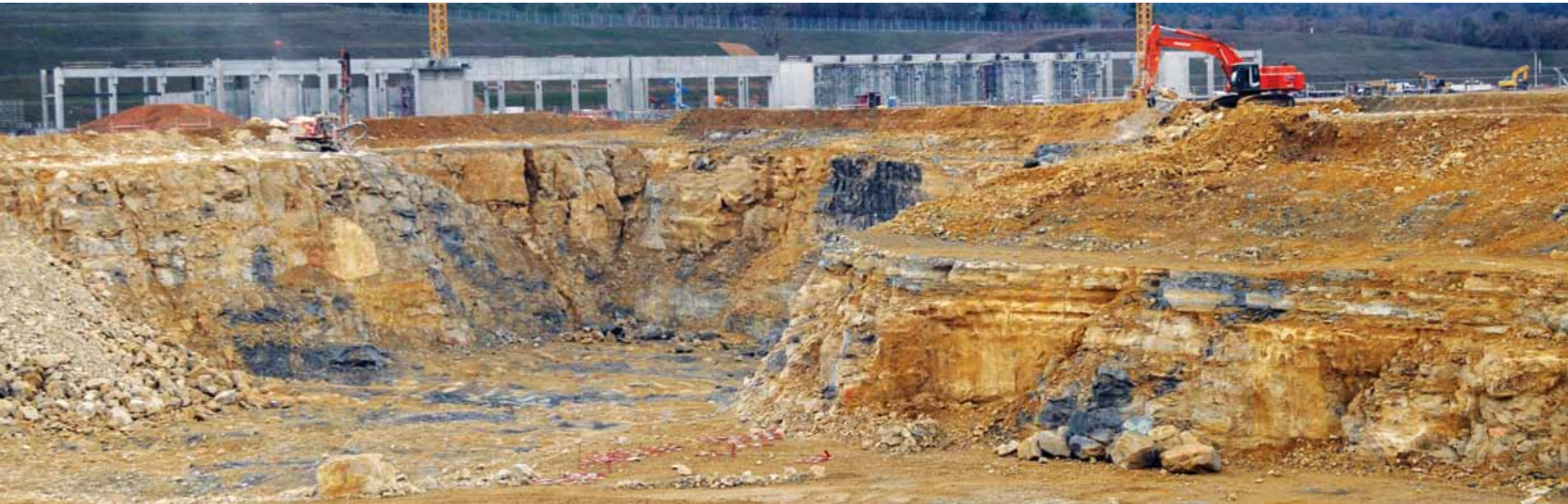
Across the excavation worksite in December 2010, the first concrete pillars of the Poloidal Field Coils Winding Facility are seen in the distance. Photo: F4E
